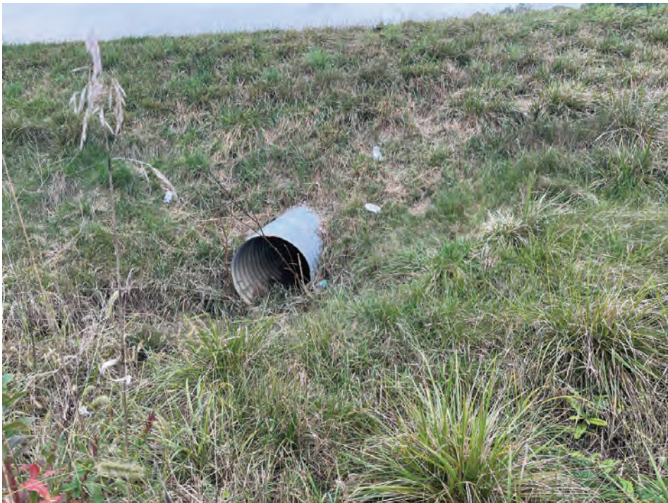
19. Looking W towards the small structure on the E side of SR 1 (10/6/2021)
