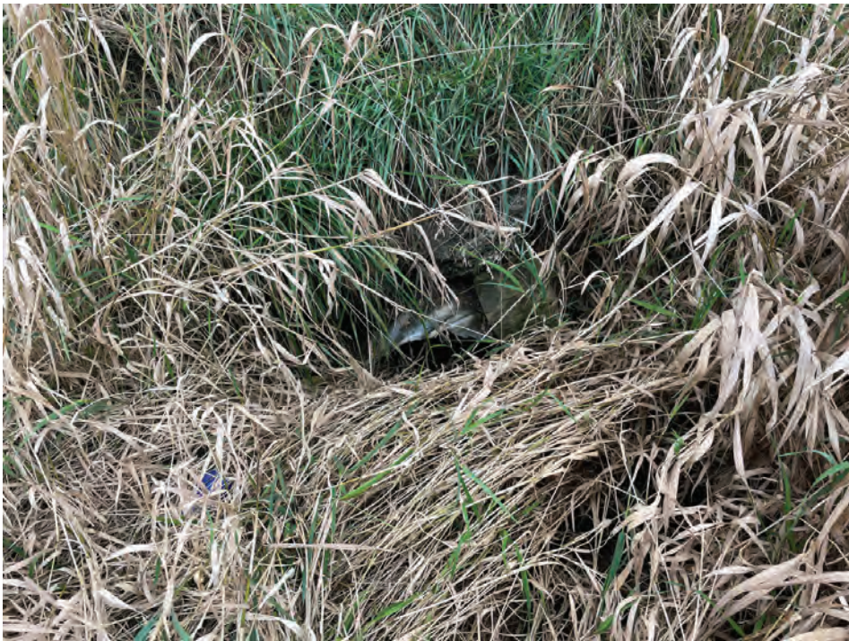
33. Looking W at the small structure inlet on the E side of SR 1 (10/6/2021)
