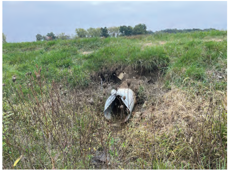
18. Looking E towards the small structure on the W side of SR 1 (10/6/2021)
