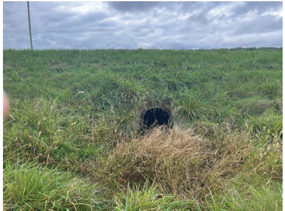
74. Looking W at towards small structure inlet on E side of US 27 (10/15/2021)
