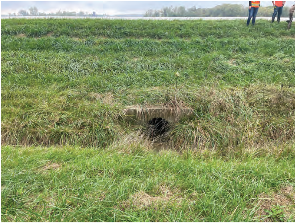
53. Looking W towards the small structure on the E side of US 27 (10/15/2021)
