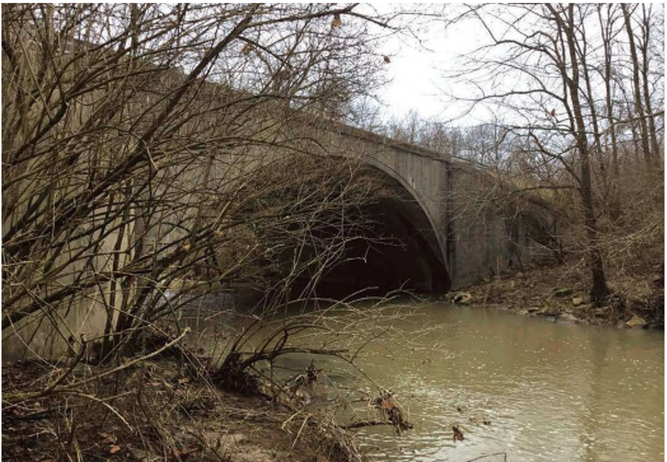
14 Looking northeast at “Contributing” reinforced concrete arched bridge [Bridge No. 046-16-00945 / NBI No. 17400] (RQAW #3) carrying SR 46 (Main Street) over Muddy Fork Sand Creek.
