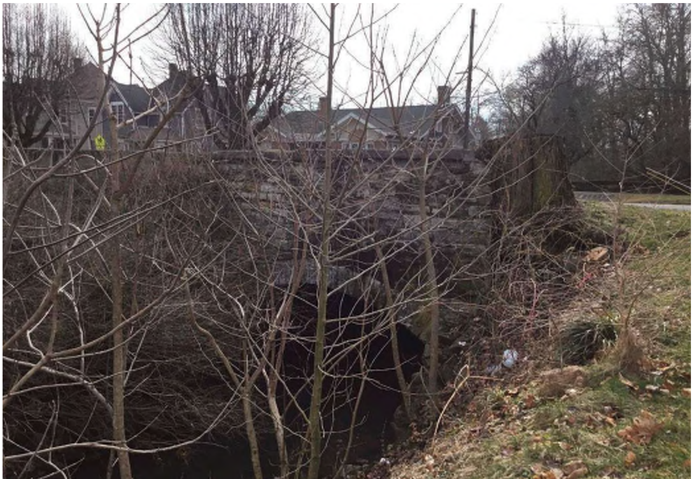
60. February 2020 photo looking southeast at stone arch bridge, a “Contributing” structure to the Greensburg Eastside Residential Historic District. The bridge was replaced in the summer of 2020.
