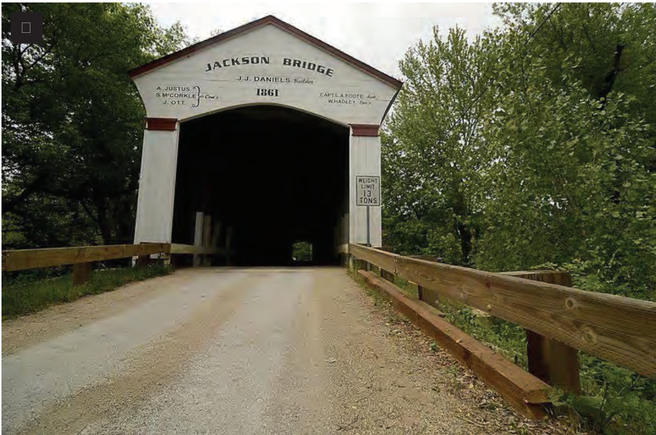
Tribune-Star/Joseph C. Garza Damage to the support beams: A broken support beam sits under a guard rail at the Jackson Bridge near Bloomingdale in Parke County on Wednesday.
