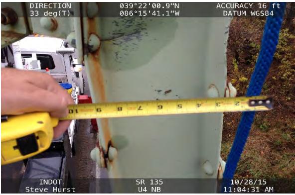
Crack at Sway Bracing L4U4 East Truss Facing North 1
