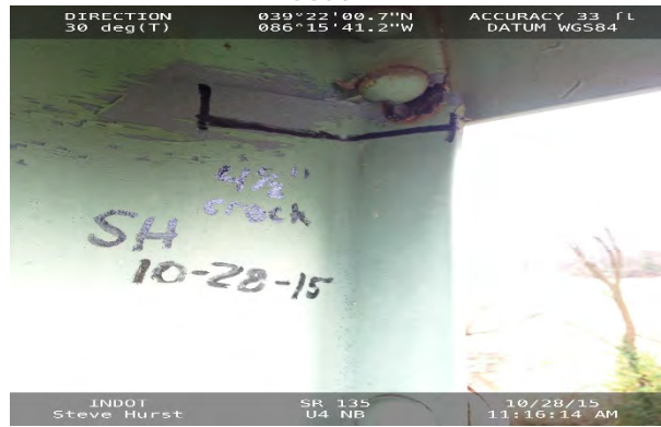
Crack at UC L4U4 East Truss facing South
