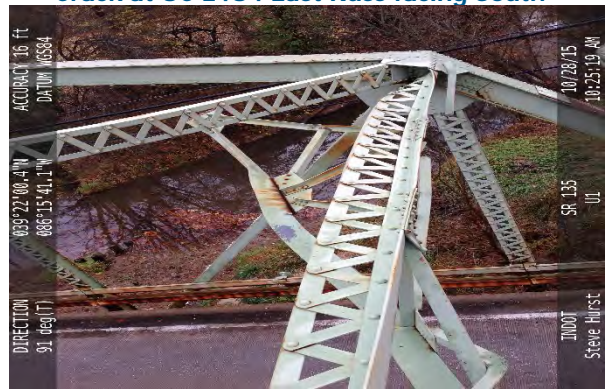
Damage to Sway Bracing South Portal Facing East
