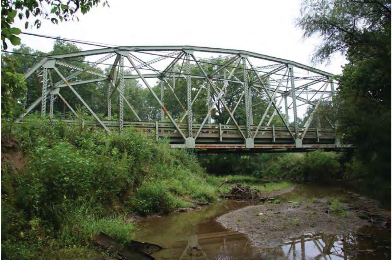
Bridge before recent collision & damage
