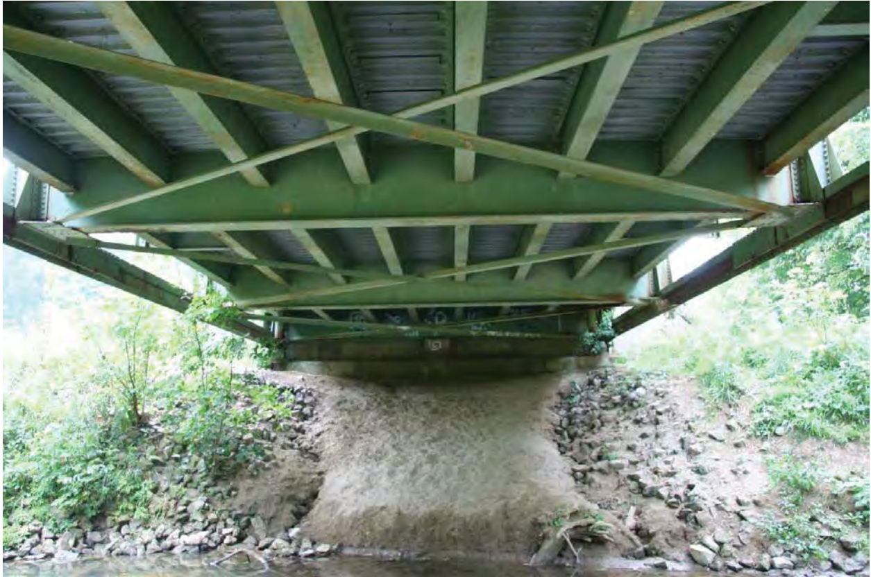
Bridge before recent collision & damage
