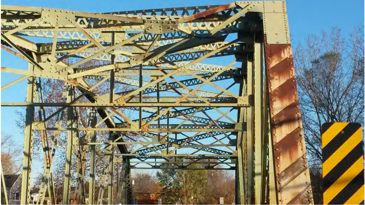
Damaged south portal – before
