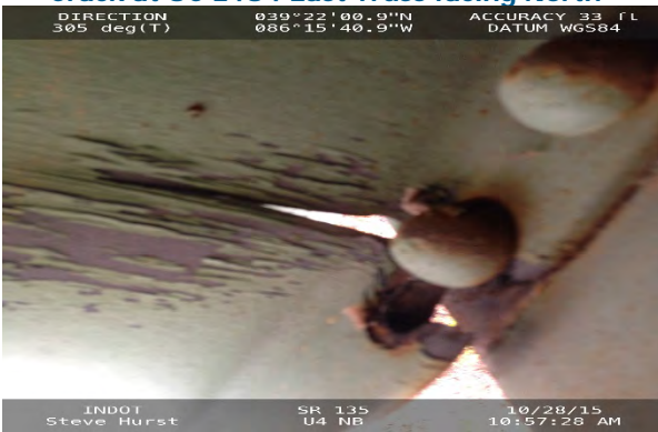
Crack close up at UC L4U4 East Truss facing North
