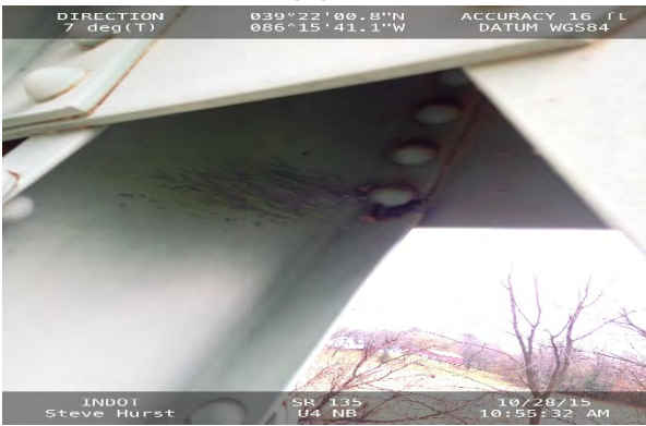
Crack at UC L4U4 East Truss facing North
