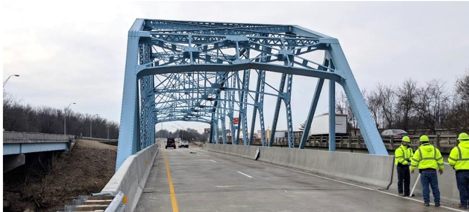
Figure 2-1: Bridge strike on Bridge No. 41-82-03286 HSBL (NBI No. 014310) by an off-route overheight vehicle.
