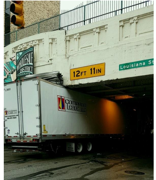
Figure 3-1: Bridge strike with static signage. Bridge shown carries Union Station railroads tracks over S Meridian Street in downtown Indianapolis. Note that after this photo was taken, flashing beacons were added to this bridge crossing.
