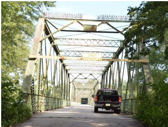
Figure 4-4: Vertical clearance bar constructed at entrance of CR100E over Wabash River bridge in Warren County, IN.
