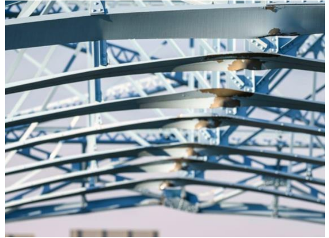
Figure A-0-1: Damage to the US 41 Through-Truss Bridge Portals.
