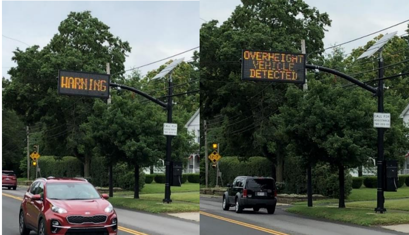
Figure 5-3: Dynamic Message Sign with warning message.
