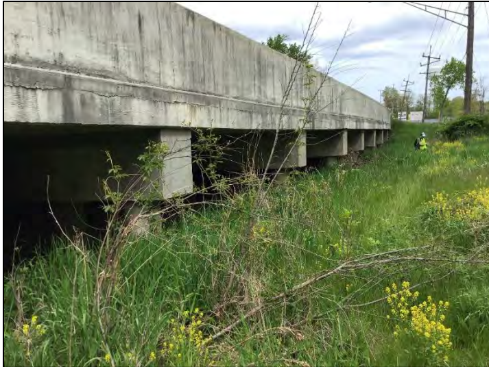
Photo 1. East side of bridge over Muck Pocket ((6)51-45-01943 B) and Wetland A, viewing north, 5/17/2021
