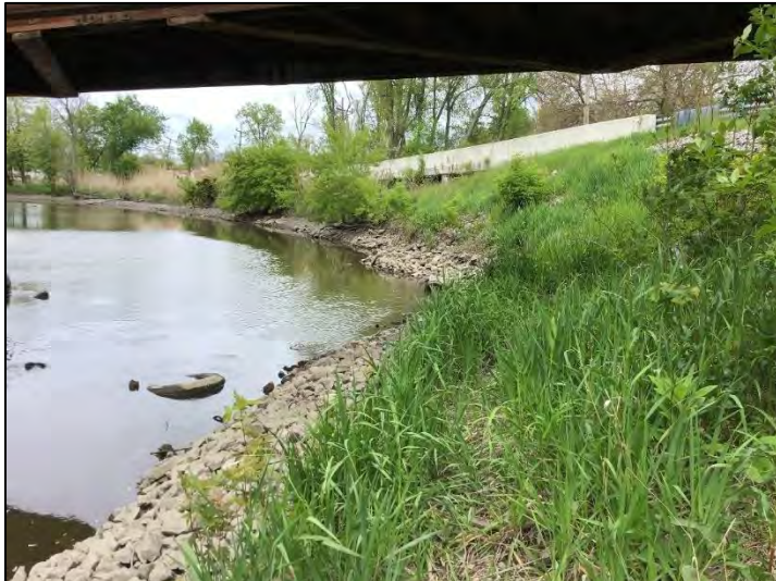
Photo 7. Bank of Deep River on west side of bridge over Muck Pocket ((6)51-45-01943 B), viewing northeast, 5/17/2021
