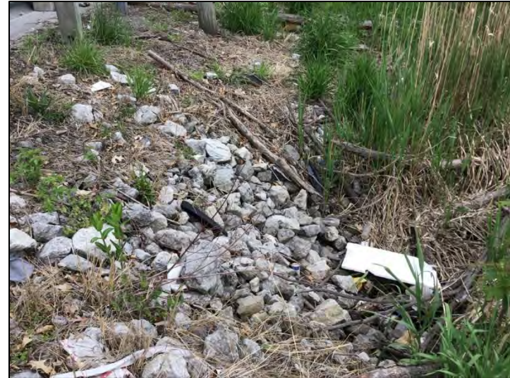
Photo 10. Presumed location of Str. 2 outlet on northwest side of the bridge over Muck Pocket, viewing south, 5/17/2021
