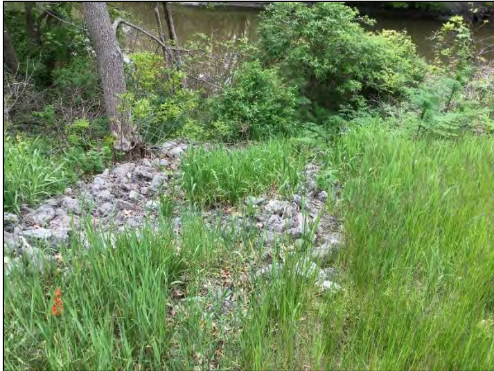
Photo 9. RSD 2 on southwest side of the bridge over Muck Pocket, viewing west, 5/17/2021
