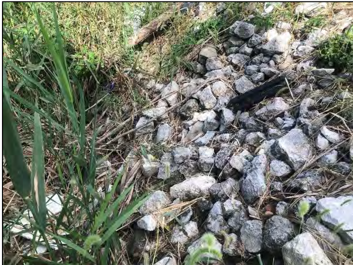
Photo 55. Presumed outlet of Str. 2 north of bridge over Muck Pocket, viewing north, 9/25/2021
