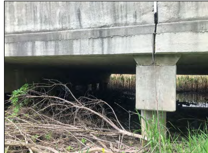
Photo 16. Open Water 2 under bridge over Muck Pocket ((6)51-45-01943 B) with standing water, viewing west, 5/17/2021
