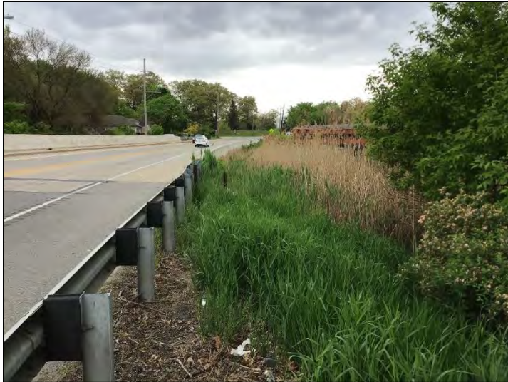
Photo 21. West side of bridge over Muck Pocket ((6)51-45-01943 B) and Wetland C, viewing south, 5/17/2021
