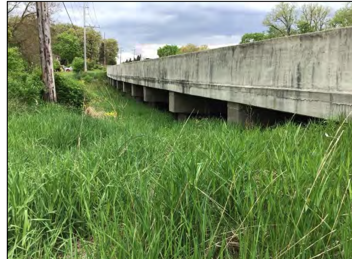
Photo 4. East side of bridge over Muck Pocket ((6)51-45-01943 B) with Wetland A, viewing south, 5/17/2021
