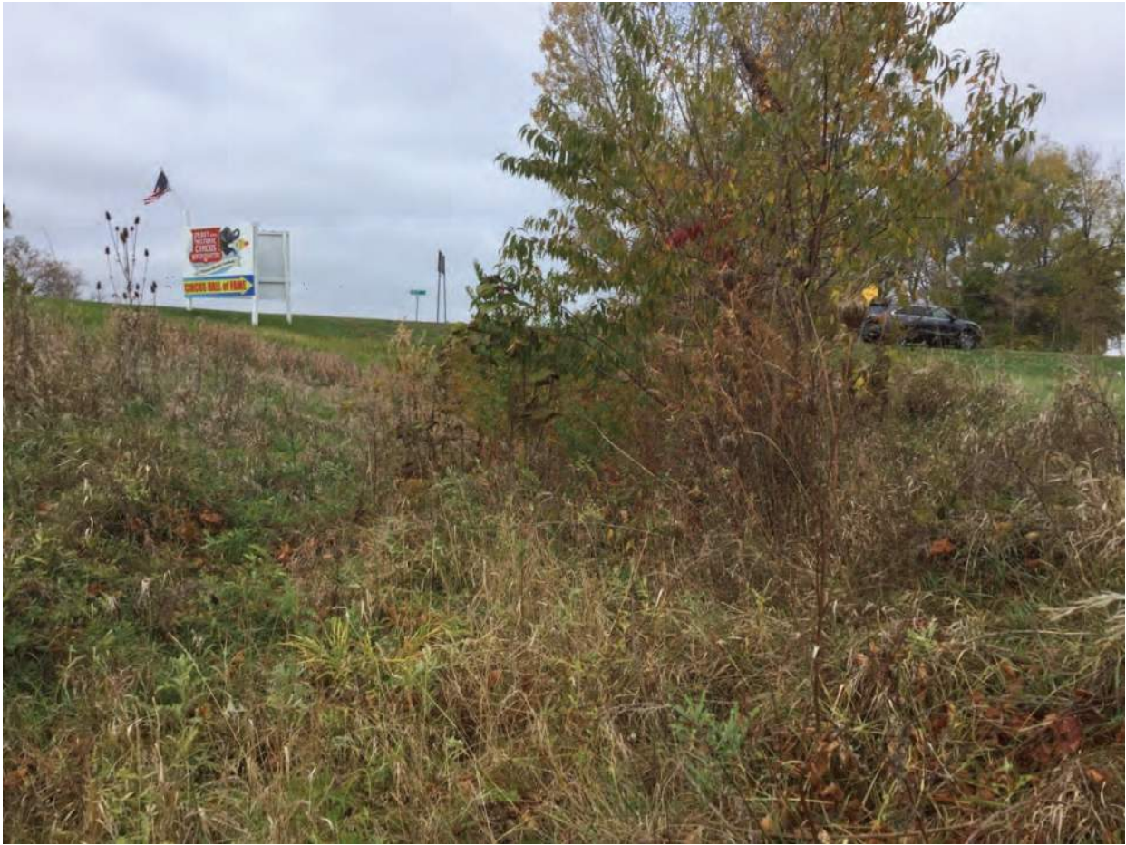
57. Looking northwest towards Circus Lane and culvert COID 19925 from RSD 1, looking towards riprap lined portion of ditch
