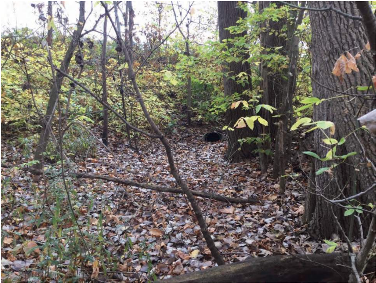
61. Looking east towards Circus Lane culvert COID 19925 from where RSD 1 intersects UNT 2 to Mississinewa River
