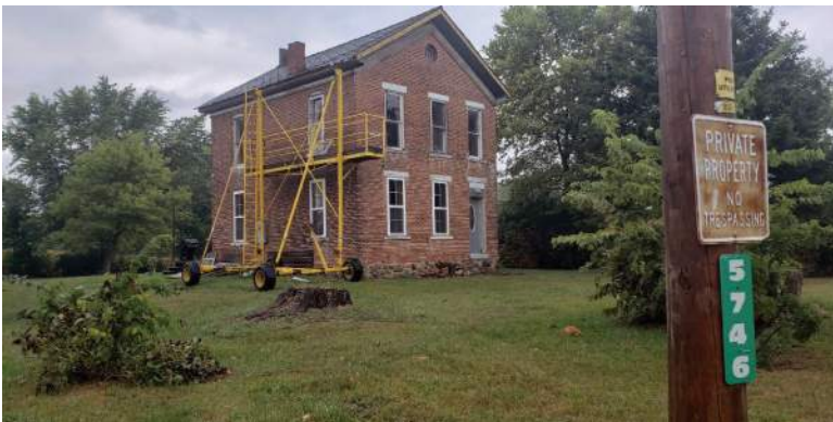
B. Looking northeast to 5746 SR 124 which is a 2 story brick house undergoing renovation
