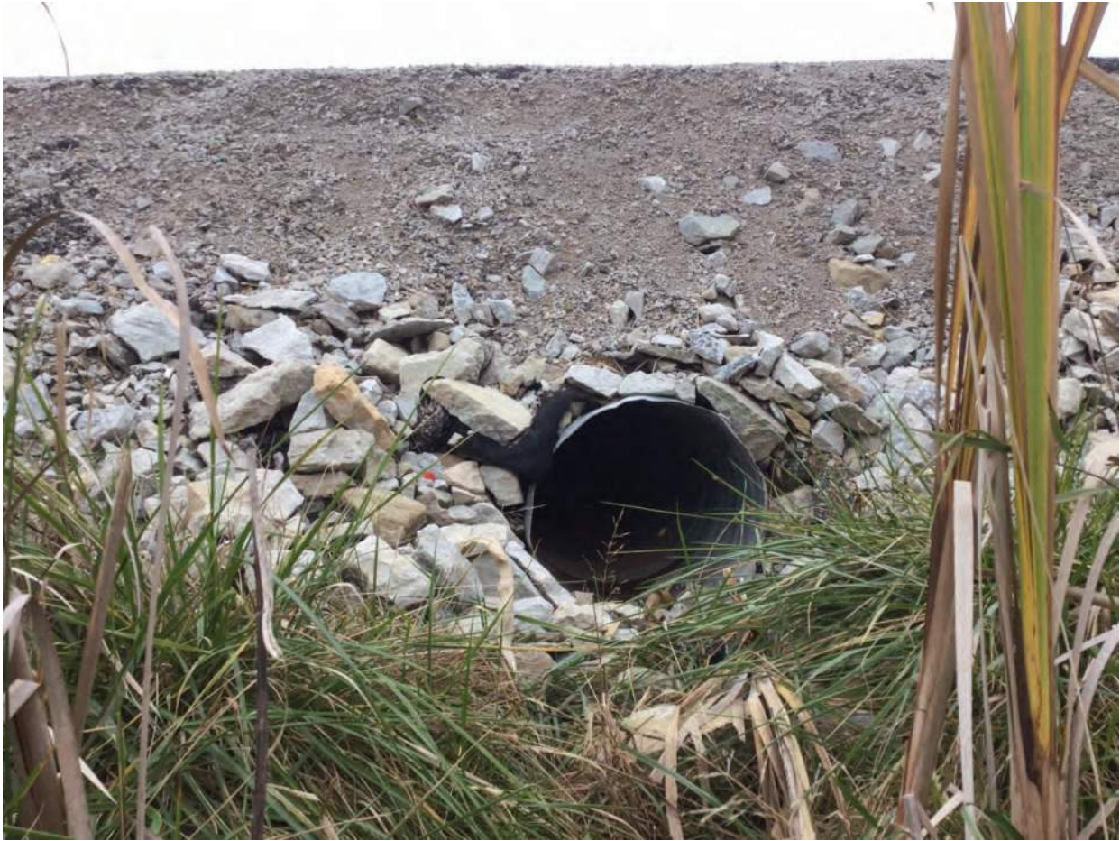
85. Looking west to culvert COID 19871 from UNT 1 to Asher Branch and Wetland A
