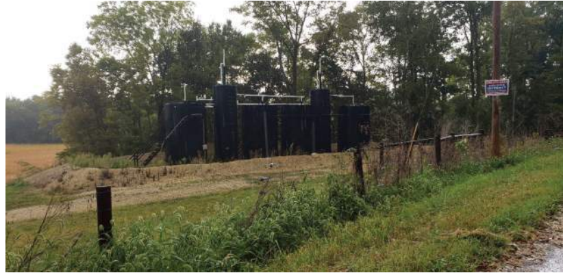
C. Looking northeast at above ground petroleum storage tanks
