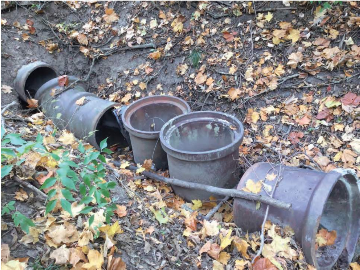
51. Looking north at failed pipe conveying UNT 1 to Mississinewa River
