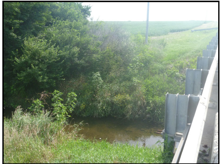
Photo 20 – Northeast Quadrant of Crossing: Facing northeast toward the northeast bank of Greenwood Ditch at the SR 18 bridge.
