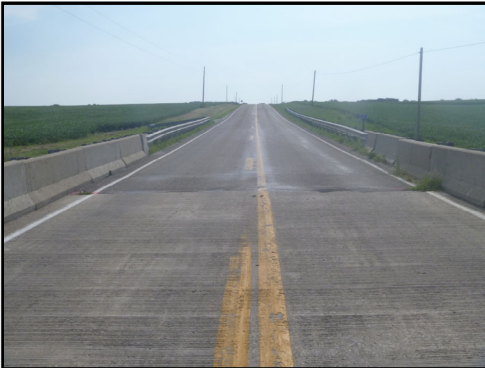
Photo 25 – SR 18 at Crossing: Facing east along SR 18 from the top of the bridge over Greenwood Ditch. Topography is generally flat to rolling. Creek and bridge sit in a shallow depression of the landscape.
