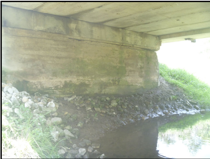
Photo 27 – Greenwood Ditch: Facing northwest toward the riprapped embankment along the west abutment of the SR 18 bridge at Greenwood Ditch.
