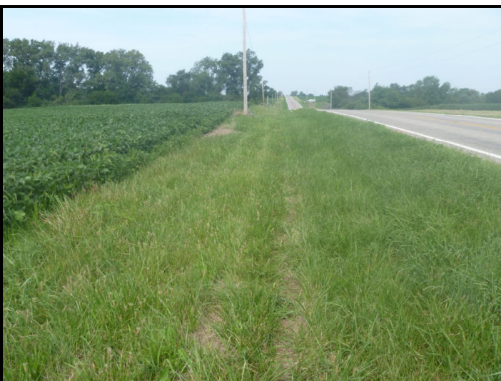
Photo 47 – Southeast Quadrant: Facing west along the south side of SR 18 near the west end of the review area. The roadside ditch is a grassy swale.
