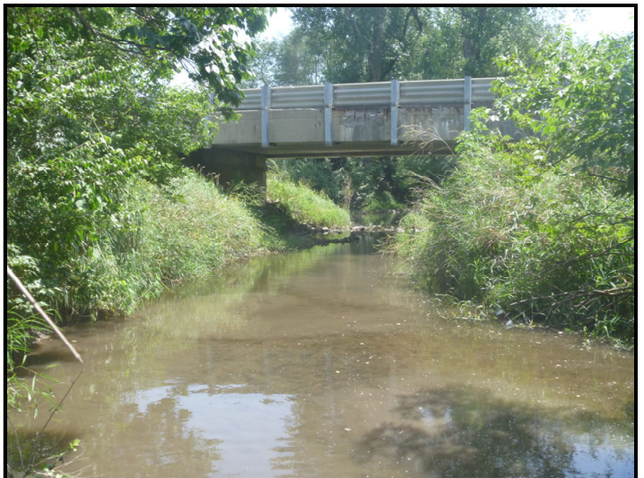
Photo 30 – Greenwood Ditch: Facing downstream to the south along Greenwood Ditch toward the SR 18 bridge, INDOT Structure No. 018-04-01689 B. The existing bridge has a single 34-foot span, with a total length of 54 feet.
