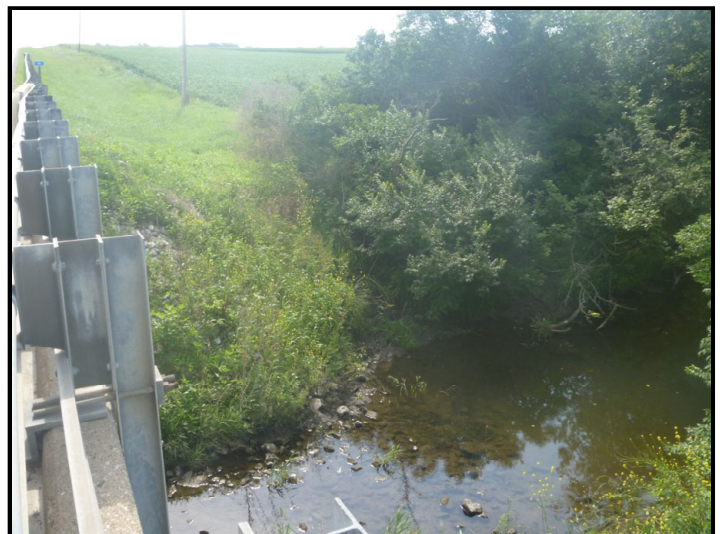
Photo 24 – Southeast Quadrant at Crossing: Facing southwest toward the southwest bank of Greenwood Ditch at the SR 18 bridge. Location of data point A-OUT in background along tree line.
