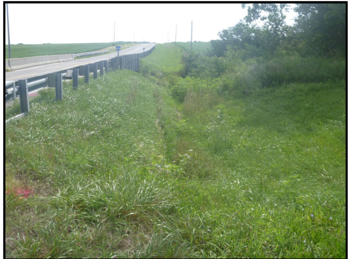
Photo 16 – Southwest Quadrant: Facing east along short vegetated roadside ditch in southwest quadrant near bank of Greenwood Ditch.
