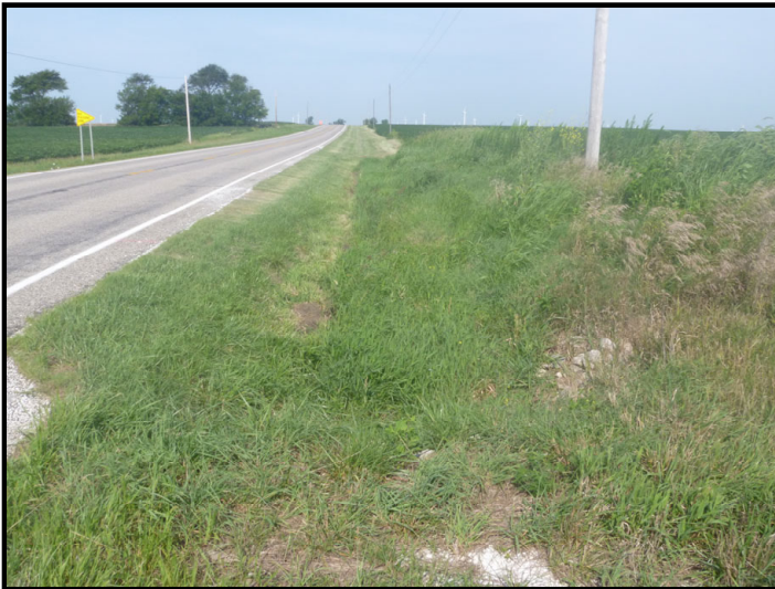
Photo 1 – RSD-1: Facing west along the north side of SR 18 beyond the review area and along the man-made roadside ditch (RSD-1).
