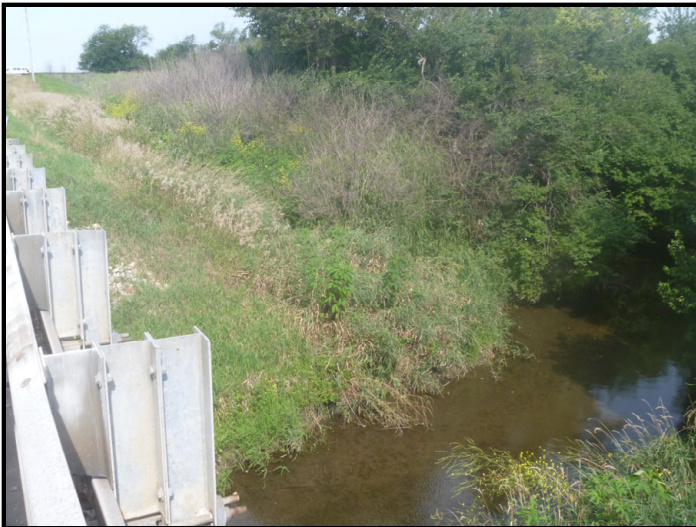
Photo 21 – Northwest Quadrant of Crossing: Facing northwest toward the northwest bank of Greenwood Ditch at the SR 18 bridge. Location of data point B-OUT in background along tree line.
