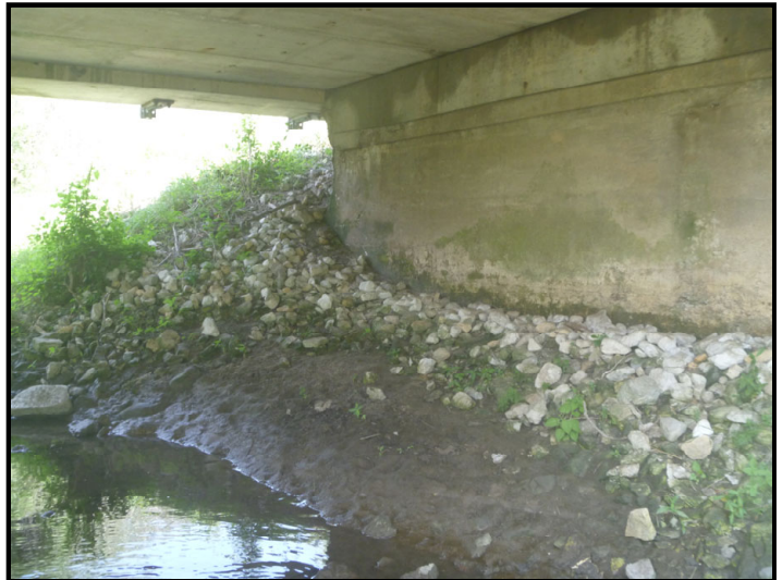
Photo 26 – Greenwood Ditch: Facing northeast toward the riprapped embankment along the east abutment of the SR 18 bridge at Greenwood Ditch.
