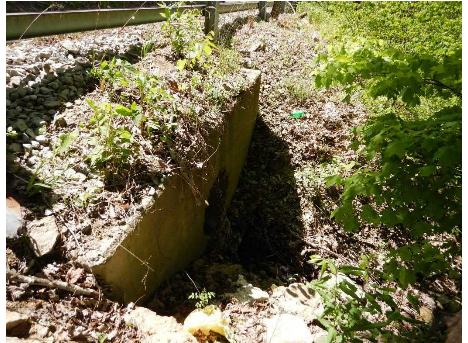
Photo 4. Facing southeast along west side of SR 7 at outlet of drainage structure.
