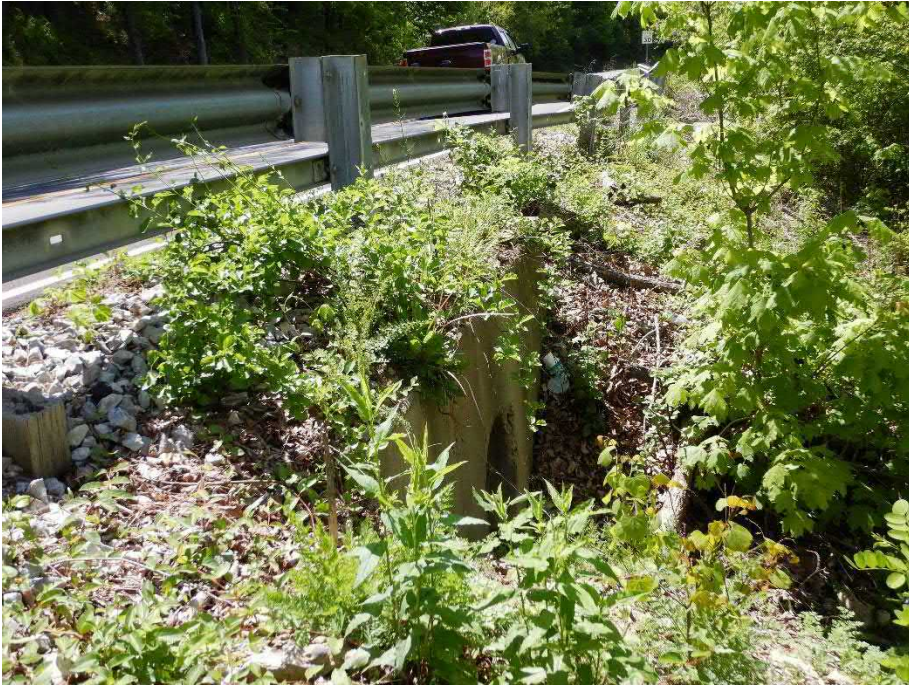
Photo 1. Facing southeast along west side of SR 7 at outlet of drainage structure.
