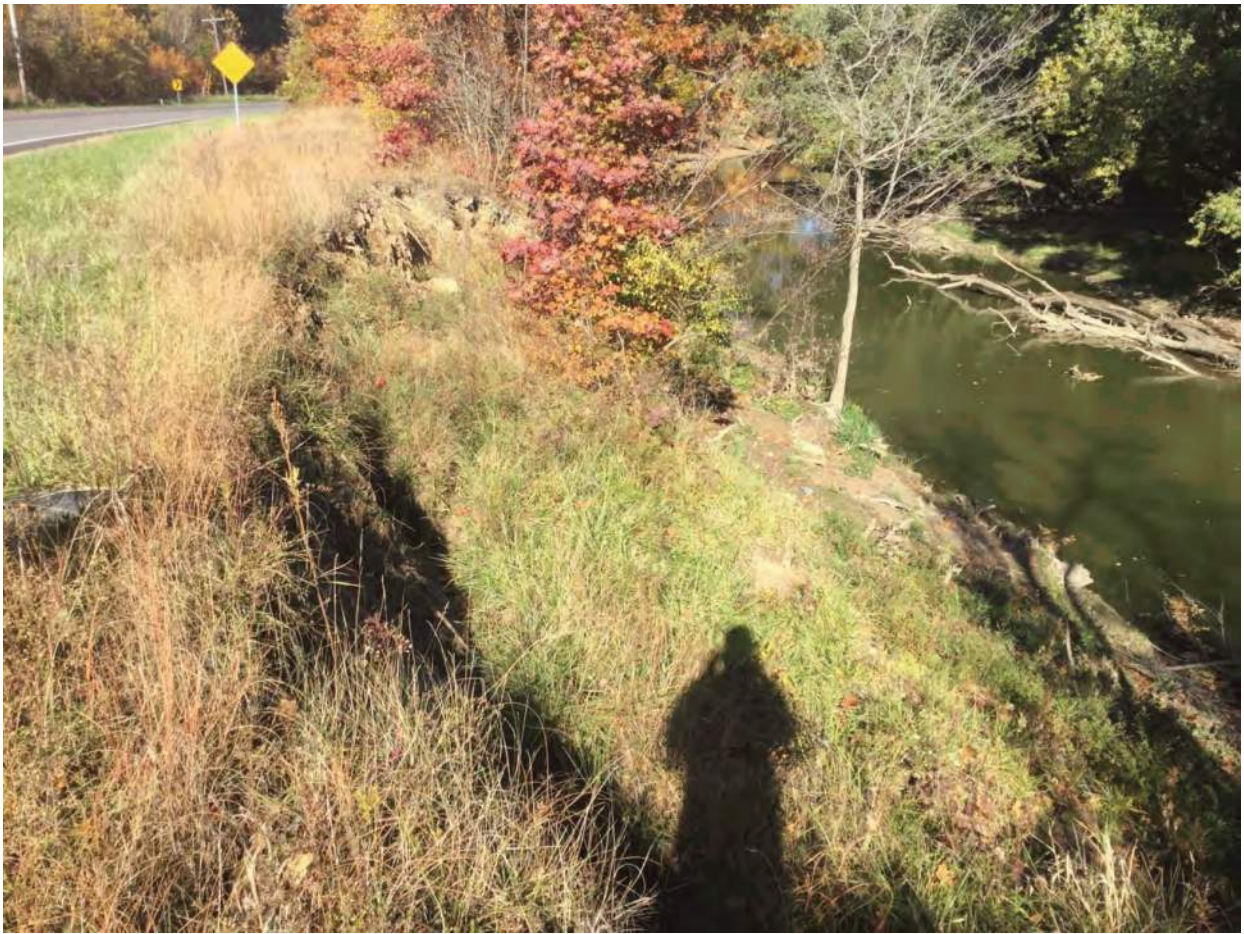
31. Looking northwest at Wabash River and SR 116 slide
