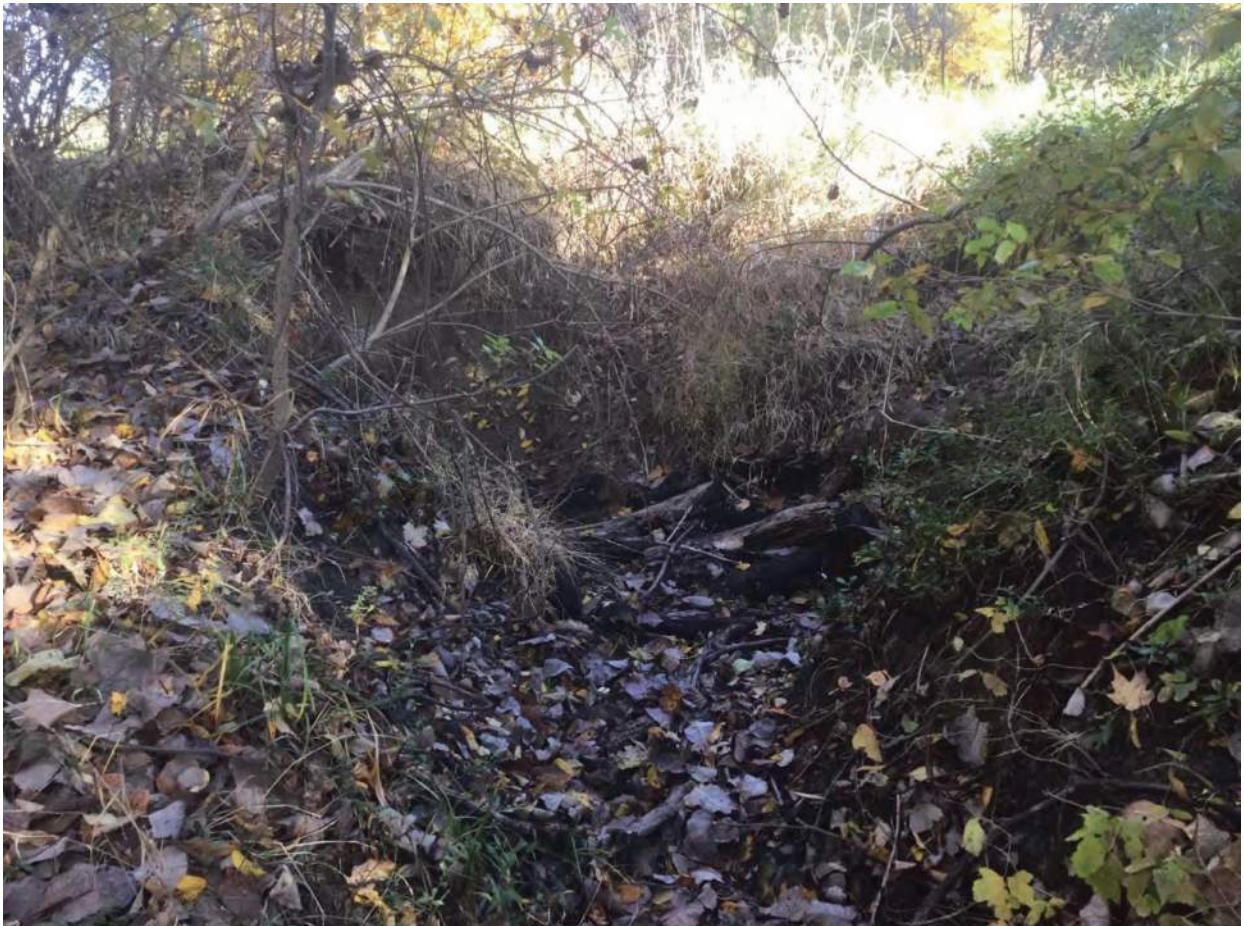
2. Looking north at erosion feature
