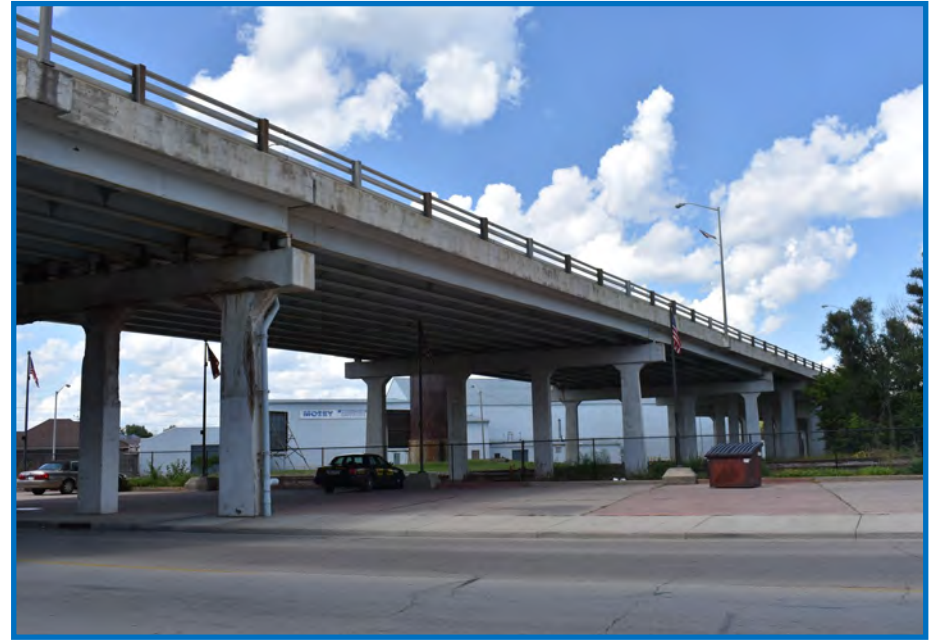
Photo 2—View of the US 27 Bridge over N. E Street and NSRR, facing northwest (09/02/2018).
