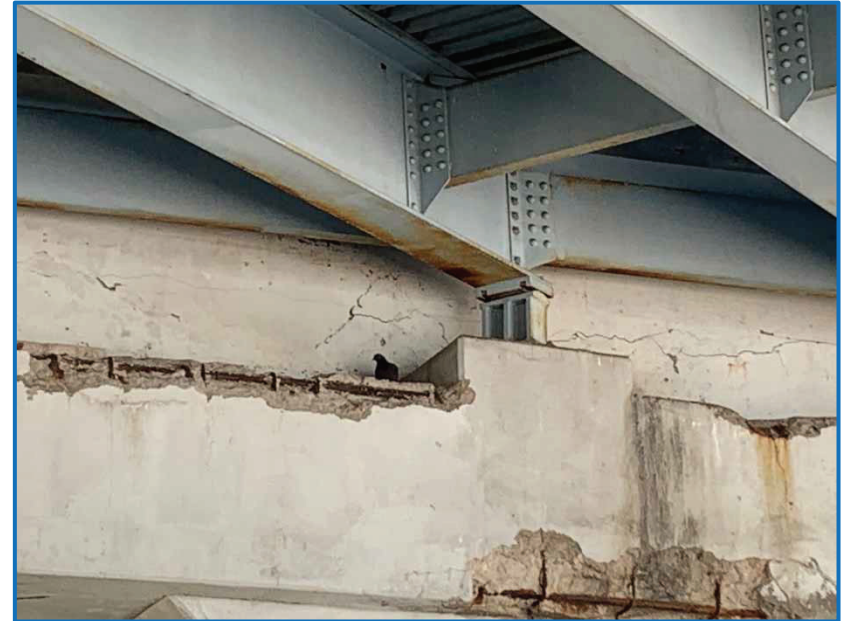
Photo 2 – View of a pigeon nesting on the US 27 bridge over North D Street (5/08/2021).
