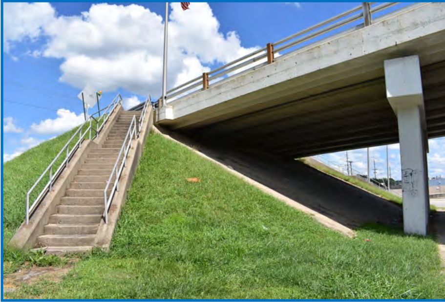
Photo 5— View of the north abutment and a staircase for the US 27 Bridge facing northeast (09/02/2018).
