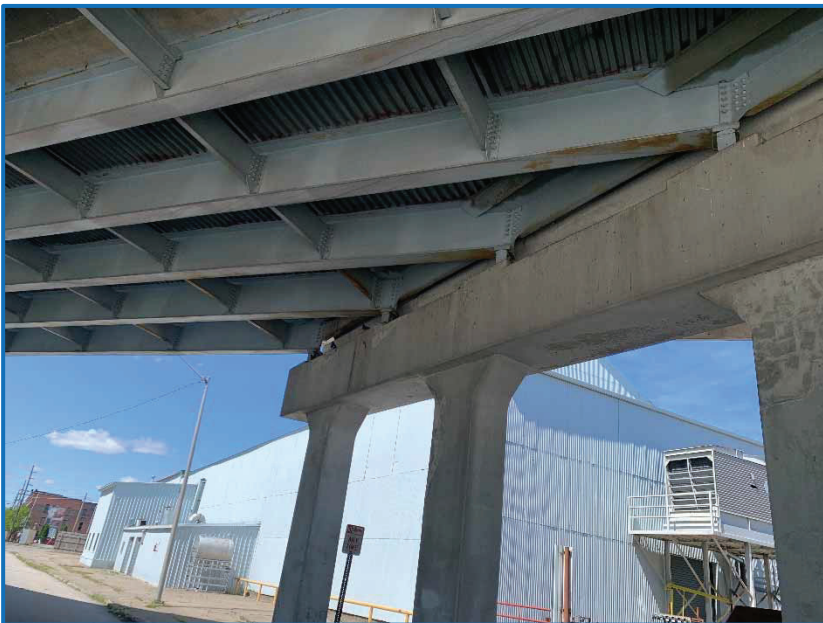
Photo 3 – View of several pigeons on the US 27 bridge on the north side of Ft. Wayne Avenue (05/08/2021).
