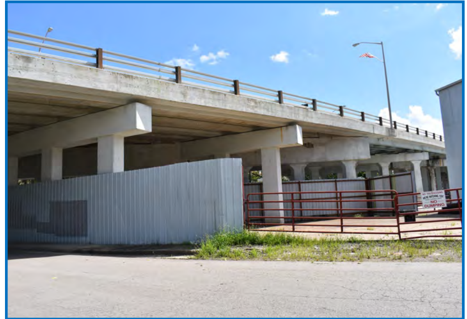
Photo 6—View of the US 27 Bridge over formerly leased property and N. F Street facing southeast. This segment of N. F Street is proposed for closure as part of this project (09/02/2018).
