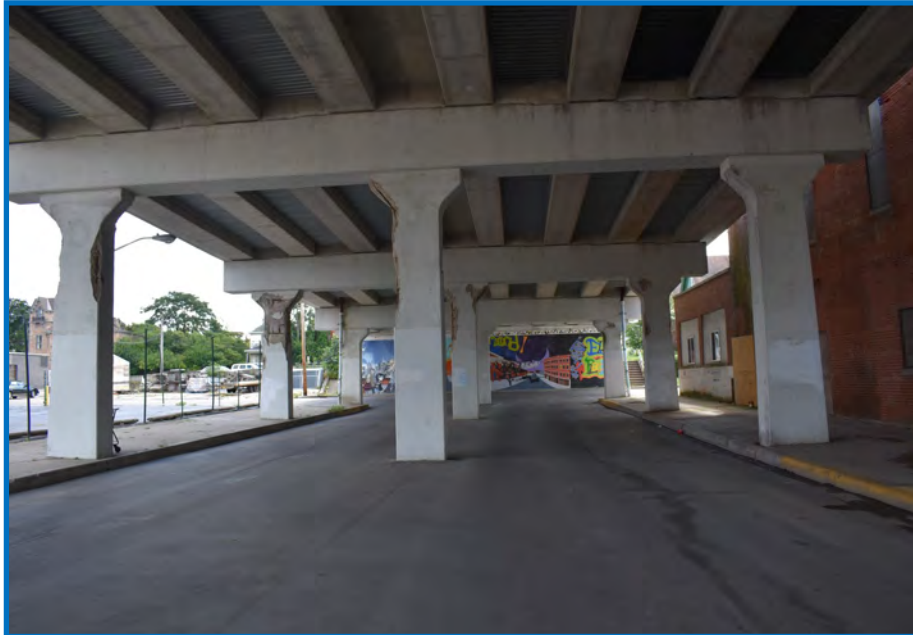
Photo 3—View beneath the US 27 Bridge at the alley that connects Elm Place and N. E Street, facing south (09/02/2018).
