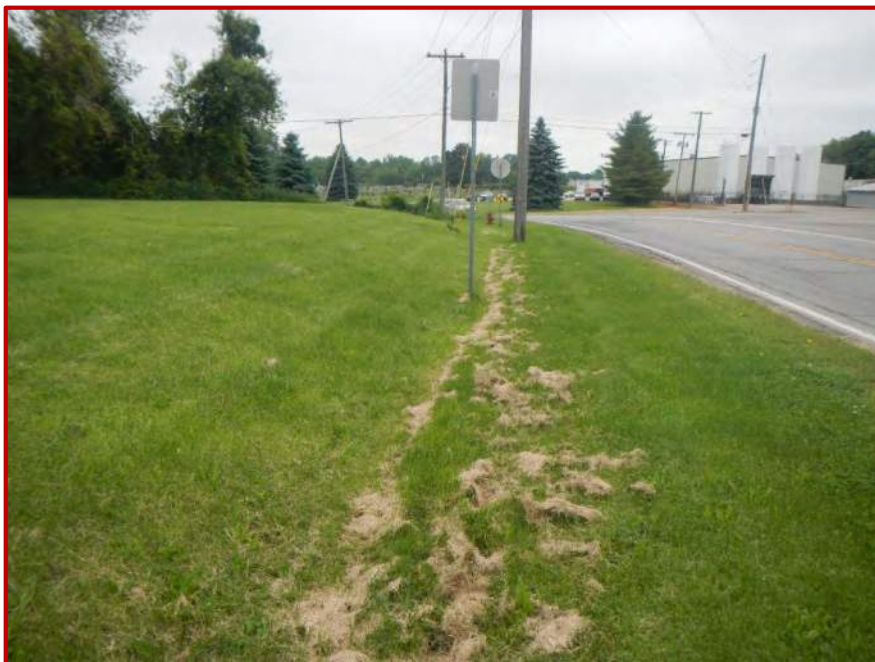
Photo 16. Looking northeast along investigated area located on the west side of SR 827 from approximately 0.01 mile north of the Broad Street.
