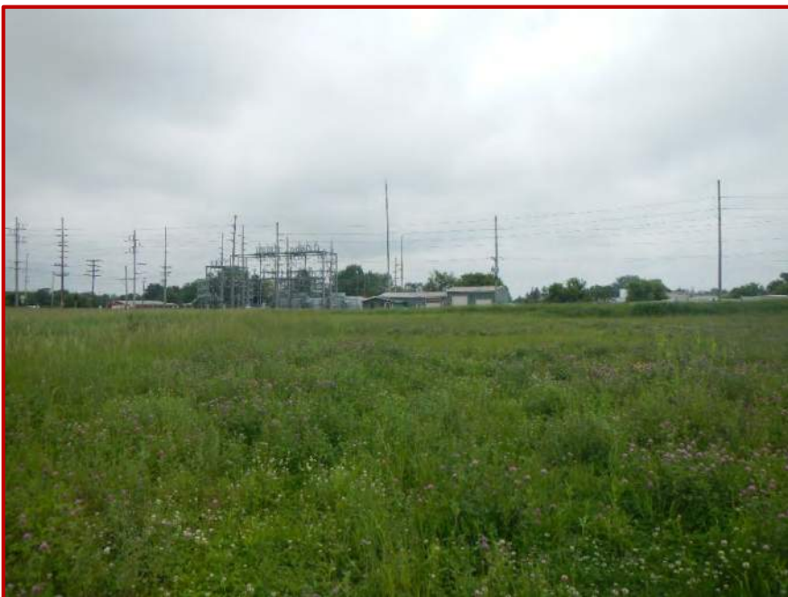
Photo 46. Looking north along investigated area located approximately 0.06 mile south of Swager Drive and 0.07 mile east of SR 827.
