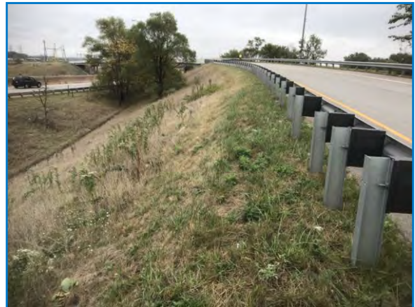
Photo 8 - View of the eastbound SR 912 exit ramp to Industrial Highway facing south (10/5/2021).
