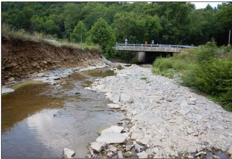
Photo 13: Looking downstream on Toddy's Branch toward SR 62. Note severely eroded bank on the river left.
