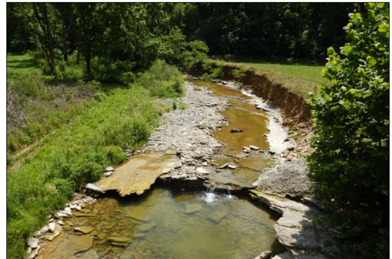
Photo 8: Looking upstream of Toddy's Branch from the Bridge carrying SR 62. Note the bedrock dominated substrate and severely eroded river left bank.
