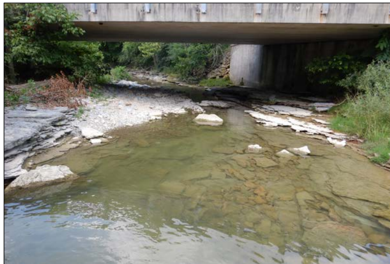
Photo 11: Looking toward SR 62 bridge from the upstream side of Toddy's Branch. Note bedrock dominated substrate.
