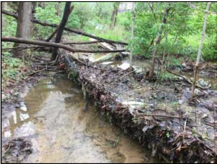
61. View of debris piling along fence in UNT 2 to Clear Creek, looking northwest.
