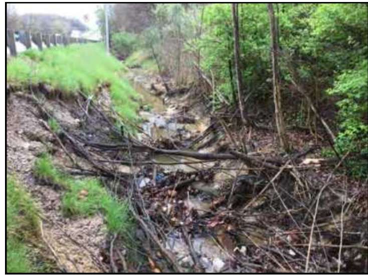
46. View of erosion along banks of UNT 1 to Clear Creek, looking northeast.
