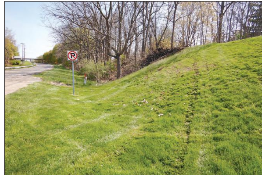
Photo 24: Roadside embankment at the toe slope of the earthen dam for Sylvan Lake, facing northeast.
