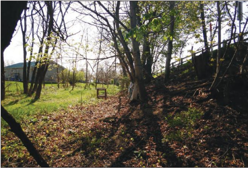
Photo 17: Embankment to the north of the east approach of the Northport Road bridge over S.R. 9, facing southeast.
