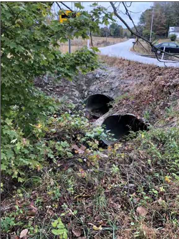
Picture 15—UNT to Kiper Creek; north view; 16 Oct 19.
