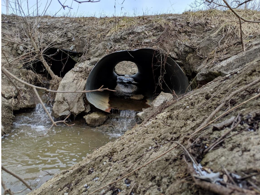
Figure 5 Bending in the existing structure.
