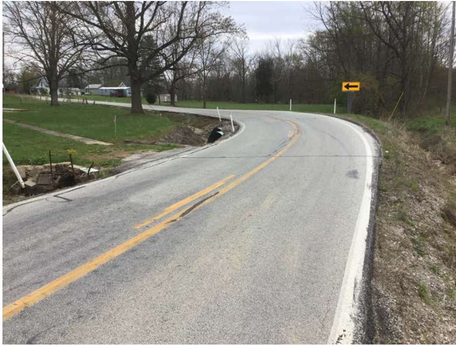
PHOTO 5 Condition Description Roadway facing South
