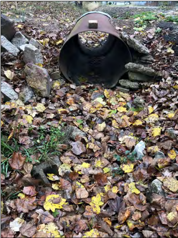
Picture 31—RSD2, southeast view; 16 Oct 19.
