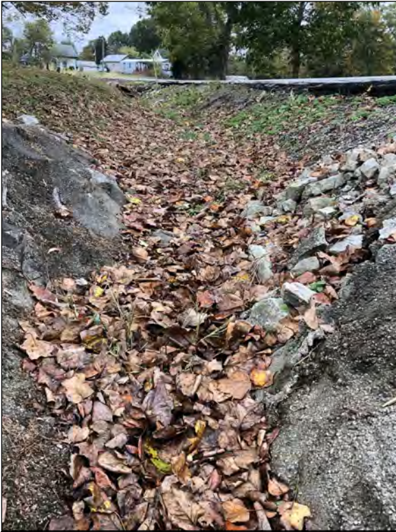
Picture 29—RSD2; southeast view; 16 Oct 19.
