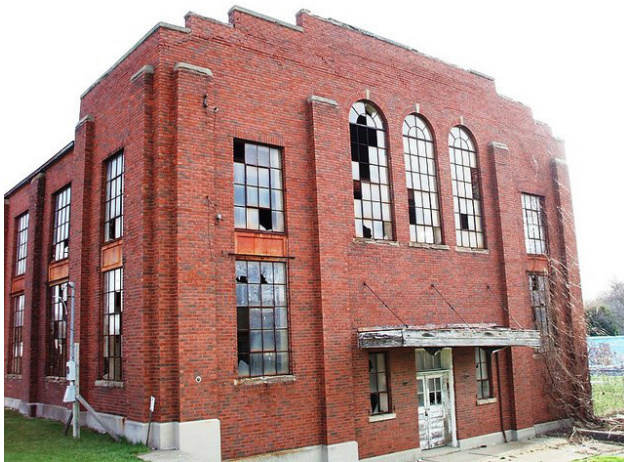
Figure 13 shows the condition of the abandoned power plant before Crossroad's Motorcycle Museum began their renovations.
