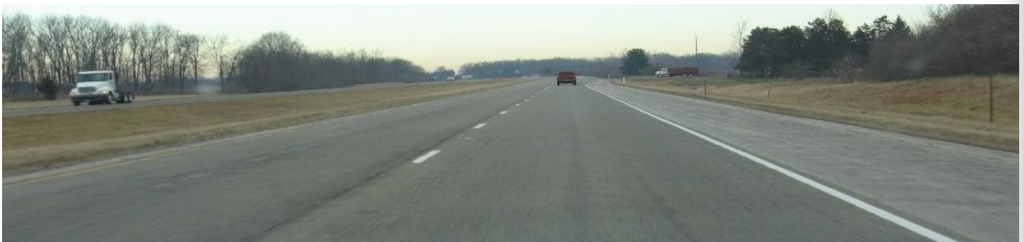
Bottom: Inspection of asphalt resurfacing of US 31 Fulton County Line to Old US 31, Kosciusko County, Indiana.
