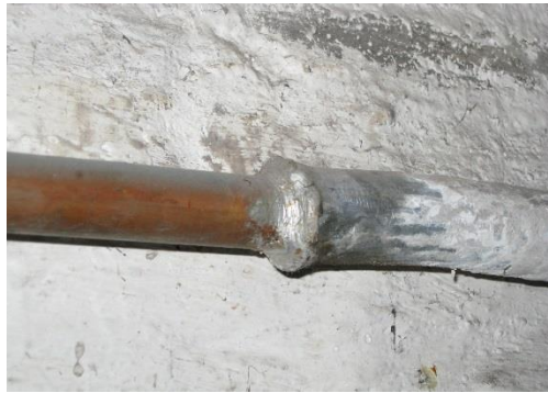
Lead Service Line (KBreker)
