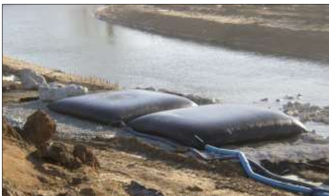
Exhibit 713.01-A. Filter bags installed on a level aggregate pad with a stabilized discharge or outflow path to the receiving stream.
