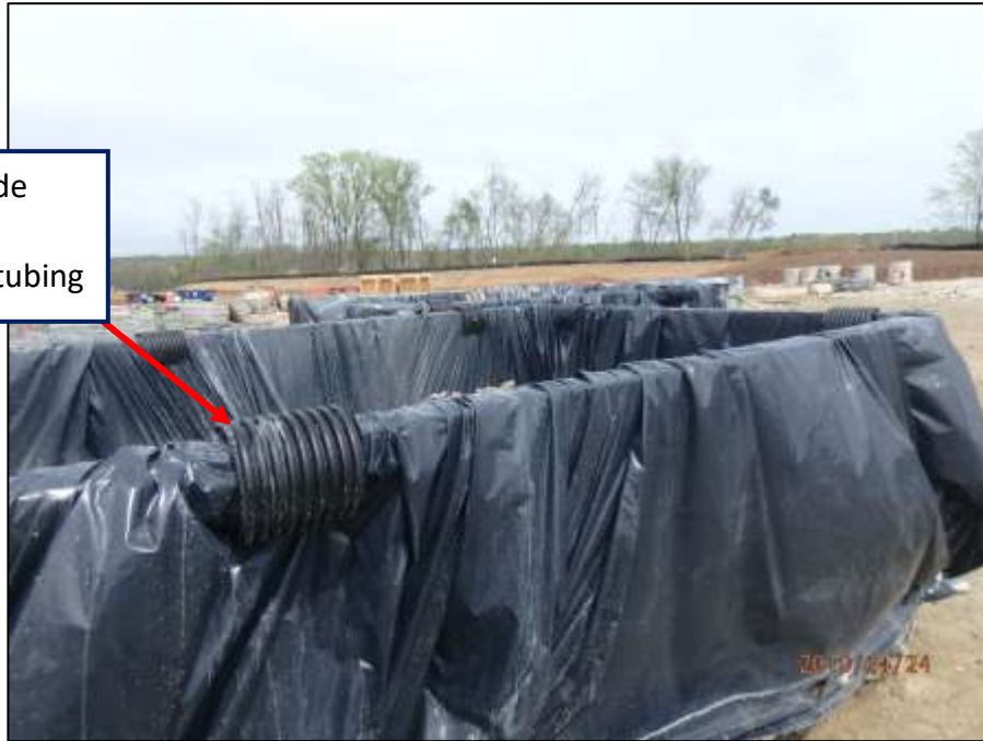
Exhibit 710.03-B. A trash dumpster has been lined with a black plastic liner to form a watertight containment for cementitious washwater. Notice the improvised clamps (sliced corrugated plastic drainage tubing) that hold the liner in place to prevent liner from sliding into the dumpster box and below the washwater and slurry pool elevation.
