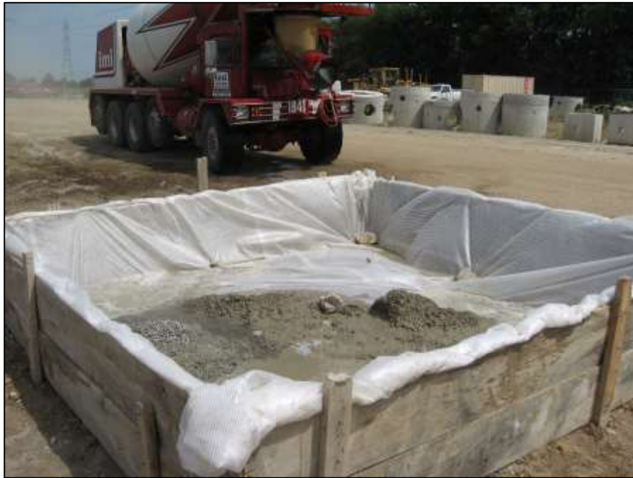
Exhibit 710.03-D. A constructed above grade wood supported washwater containment that is lined with polyethylene plastic liner.
