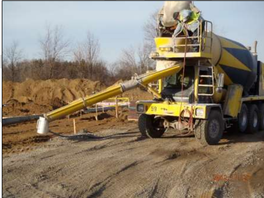
Exhibit 710.03-C. Concrete delivery vehicle using a truck mounted washwater recycling bucket that pumps the washwater from rinsing the hopper and chute back into the truck drum to return the washwater used for rinsing back to the plant for reuse or treatment. Washed aggregate can be placed on the ground or used as fill.
