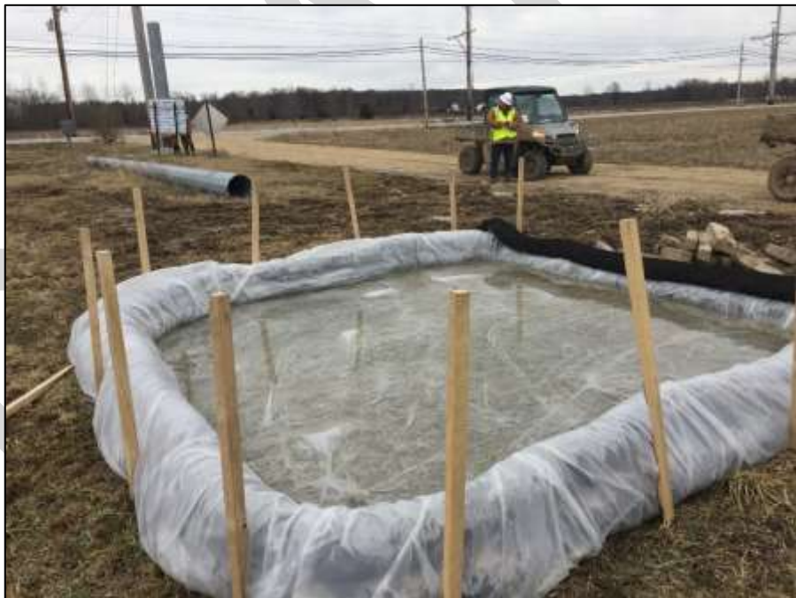
Exhibit 710.03-E. A constructed above grade washwater containment using tubular sediment controls to support the polyethylene plastic lined containment. The waterproof liner is secured from slippage into the containment by being tucked under the sediment control tubes. The wooden stakes hold the stacked tubular containment wall in place. Containment is nearly water filled and requires fluid removal to prevent overtopping from the next precipitation event.
