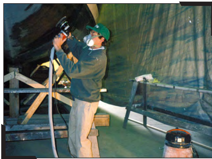
To minimize the spread of the debris, dust and paint chips, try to do all work in a covered building (Source: Jay Tanski, New York Sea Grant).
