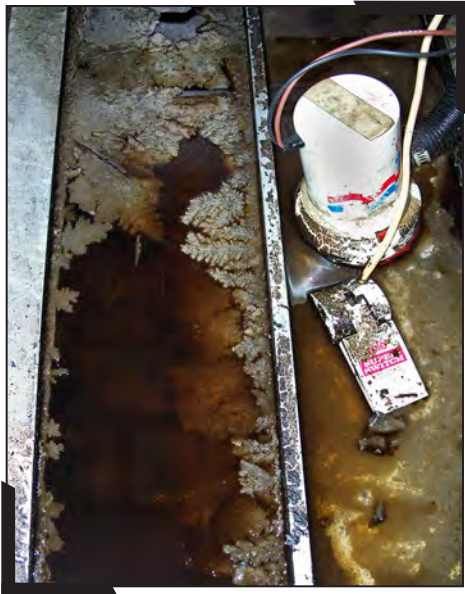
The use of a bilge sock would help prevent oil collected in the bottom of this bilge from being discharged to the lake (Photo by Joe Exl, IDNR).
