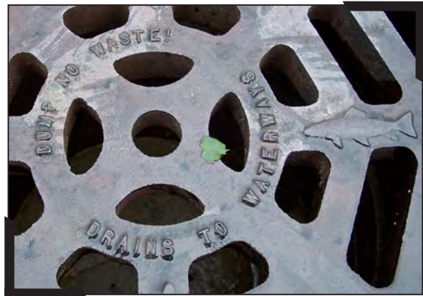
This storm drain is marked with fish symbols and text that indicates, "Dump No Waste! Drains to Waterways."
