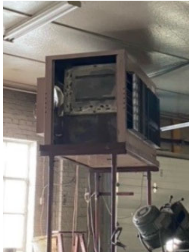
Used oil burner used for building heat
