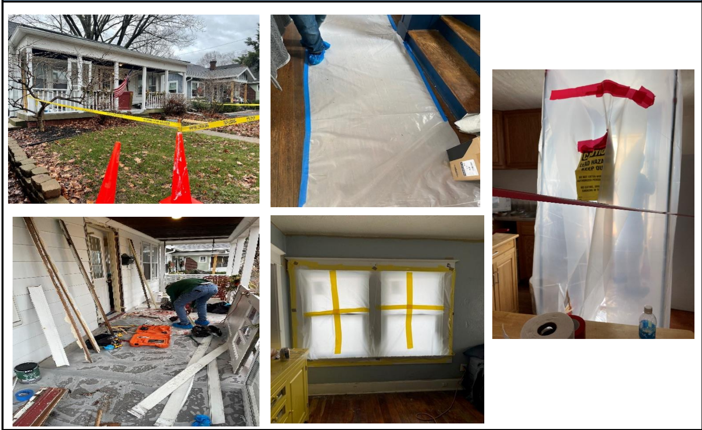
Examples of Barriers, Pathways, and Containment using 6mil Plastic Sheeting and Caution tape
