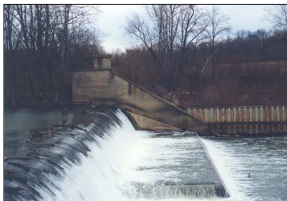
Figure 7-3 Low head, in-channel concrete dams are very dangerous due to the whirlpools, hydraulic jumps, and eddies on the discharge side.
