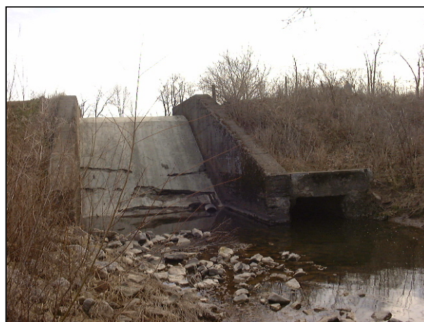
Figure 6-7 Concrete spillway showing extensive cracking and general deterioration, most likely a result of freeze-thaw effects.
