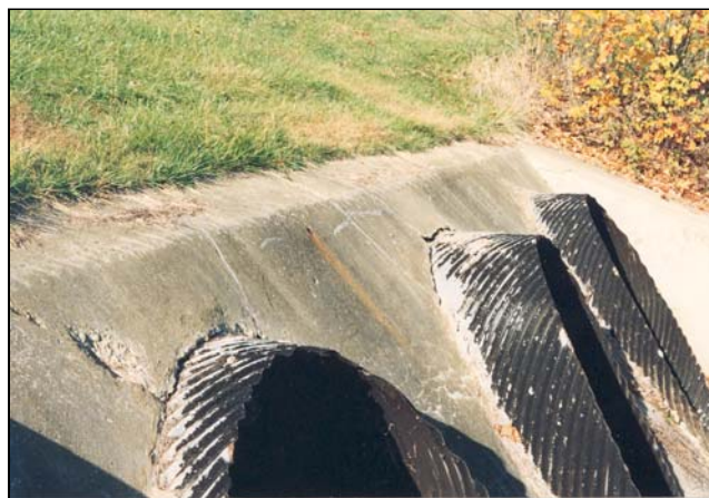
Figure 6-23 Concrete is deteriorating where these metal pipes enter a spillway riser as a result of differential expansion rates.
