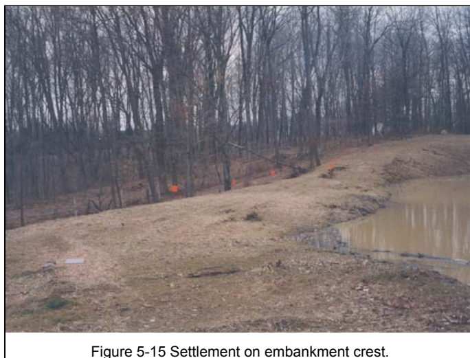
Figure 5-15 Settlement on embankment crest.
