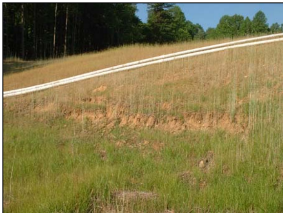
Figure 5-11 Shallow slide at toe of embankment resulting from excessive seepage and poor compaction.
