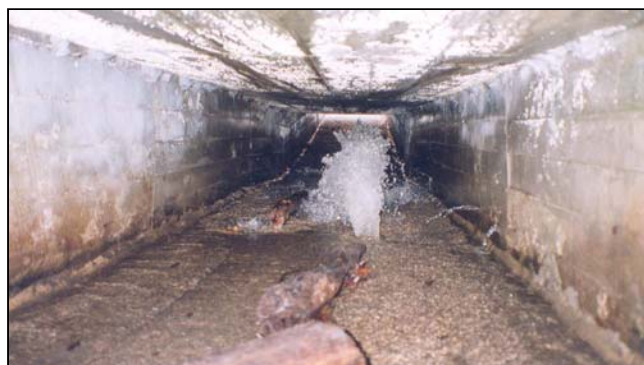
Figure 5-44 Seepage under this spillway conduit has caused piping, allowing a significant leak through conduit deficiencies.
