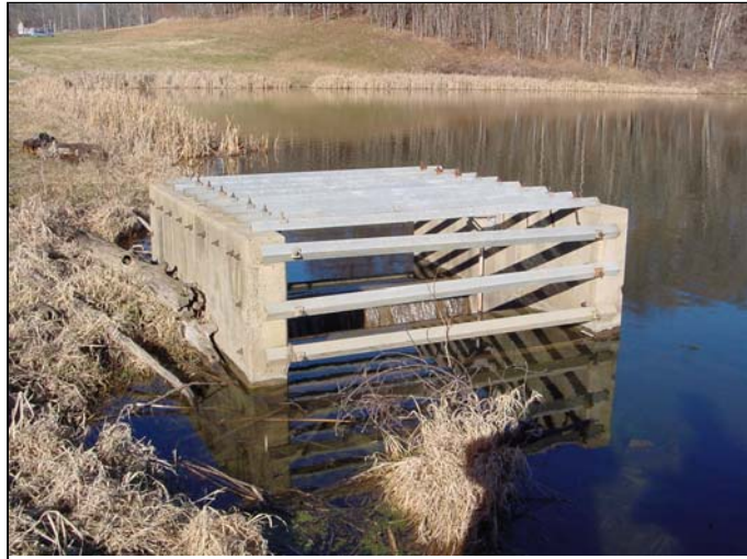
Figure 6-1 Principal spillway utilizing a riser as the control; this is the most common type of spillway in Indiana. The riser has a trash rack over the top constructed with concrete and steel bars.
