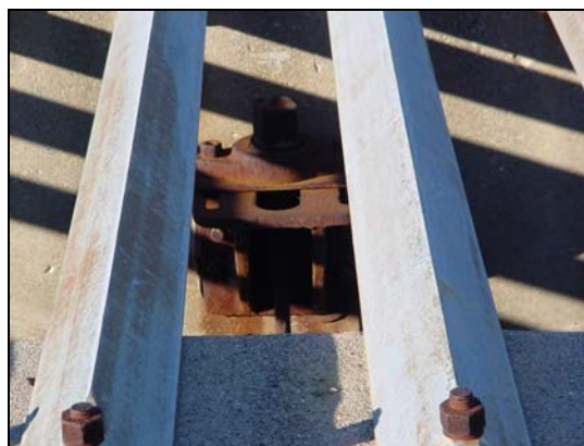
Figure 6-6 The valve stem for the outlet in this dam is conveniently located in the riser; notice the rust forming on the metal components.
