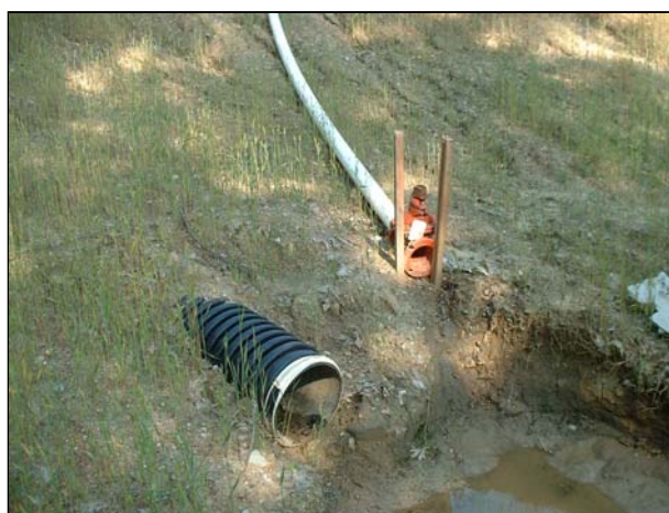
Figure 6-43 Plastic pipe used as the principal spillway; the use of this type of pipe is not recommended
