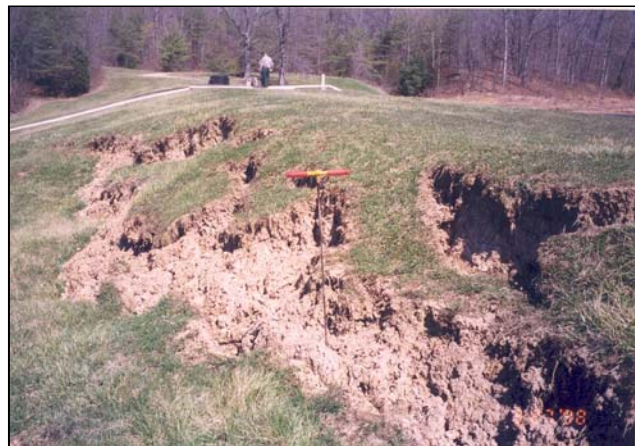
Figure 2-4 Photographic documentation of embankment slide.
