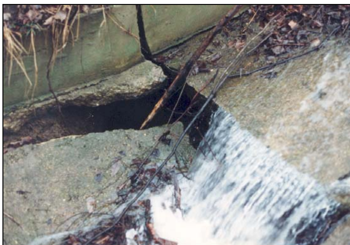
Figure 6-8 Concrete spillway with structure damage.
