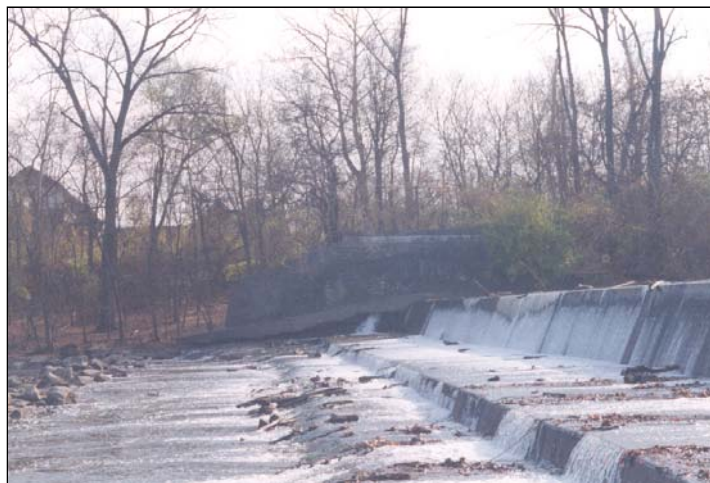
Figure 7-2 Most concrete dams in Indiana are in-channel structures that are difficult to inspect.
