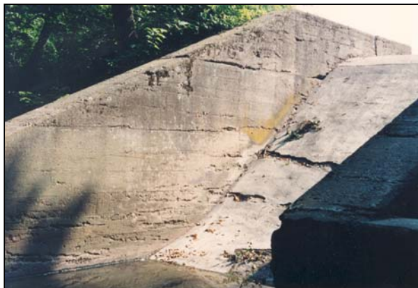
Figure 6-22 Deterioration (cracking and spalling) of a concrete spillway from weathering and freeze-thaw effects.
