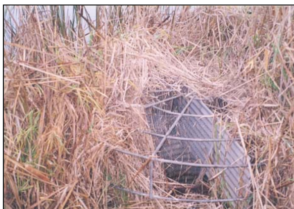
Figure 5-27 Excessive vegetation around this riser and trash rack makes visual inspection almost impossible.
