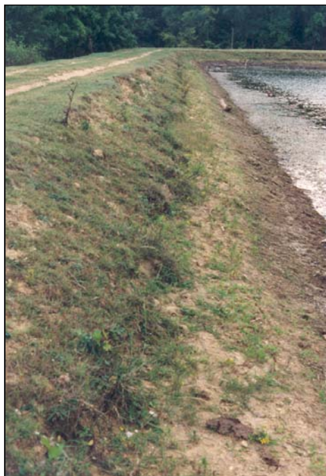
Figure 5-19 Inadequate slope protection resulting in shoreline erosion.
