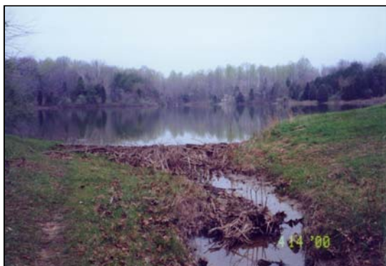
Figure 5-30 A beaver has blocked the spillway on this dam.
