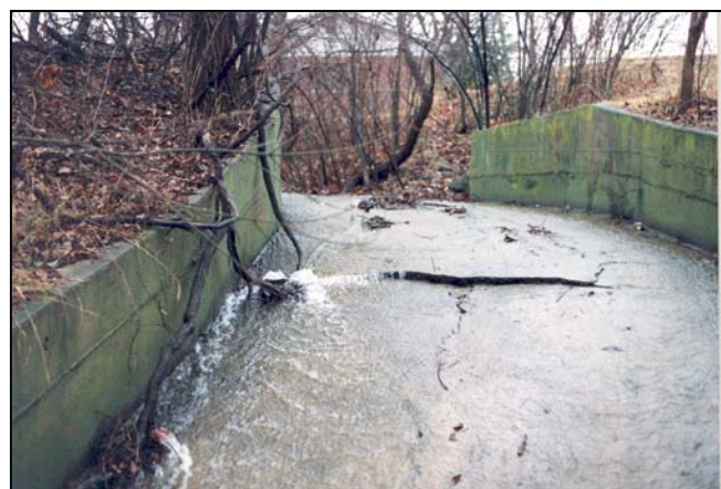
Figure 6-11 Large structural cracks with vertical displacement.
