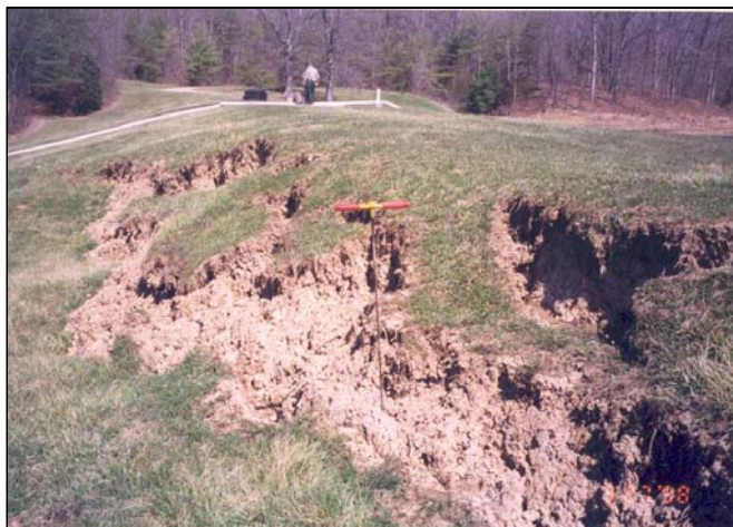
Figure 5-14 Large slide on embankment with prominent scarp.
