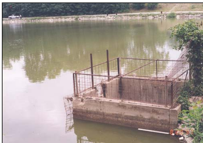
Figure 6-25 Concrete riser is spalling, exposing rebar and experiencing loss of concrete.
