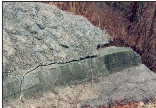
Figure 6-21 General deterioration of a concrete spillway as a result of multiple causes.
