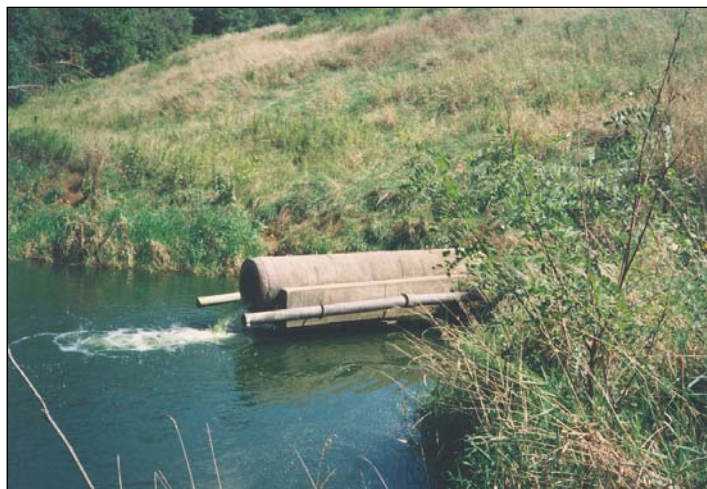
Figure 5-48 Collector pipes (beside spillway conduit) can be used to help monitor seepage through the embankment.
