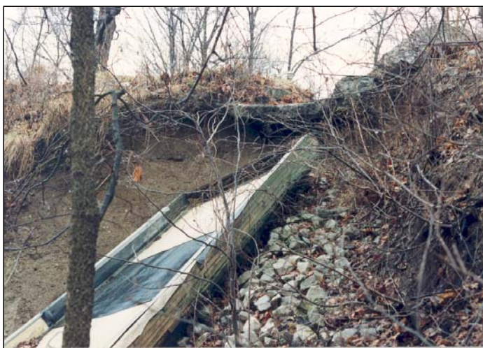
Figure 6-13 This concrete spillway was completely destroyed as a result of foundation erosion.
