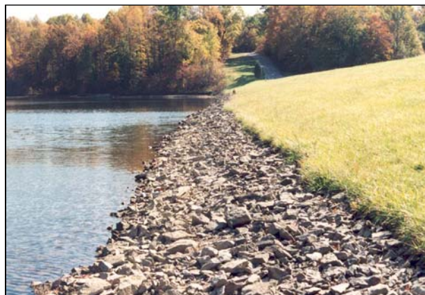
Figure 5-18 Riprap protection on the embankment slope at the shoreline, with grass on the rest of the slope.
