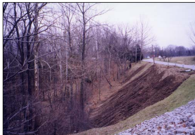
Figure 3-8 Loose fill inappropriately added to embankment slope.
