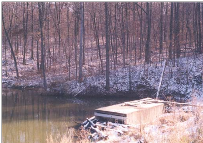
Figure 5-29 Excessive debris around the riser trash rack can reduce discharge capacity and increase water levels.
