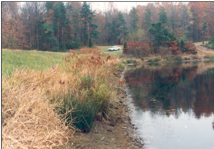
Figure 5-2 Embankment slope inspection can be hindered with excessive vegetation.
