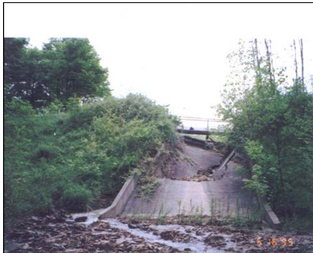
Figure 6-12 Serious structural damage requires replacement of spillway.
