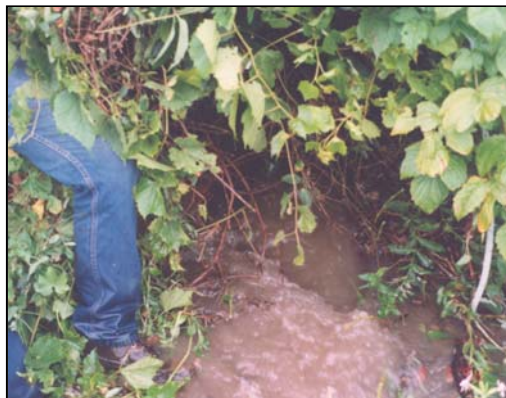
Figure 5-37 Piping through the foundation; notice the turbid discharge.
