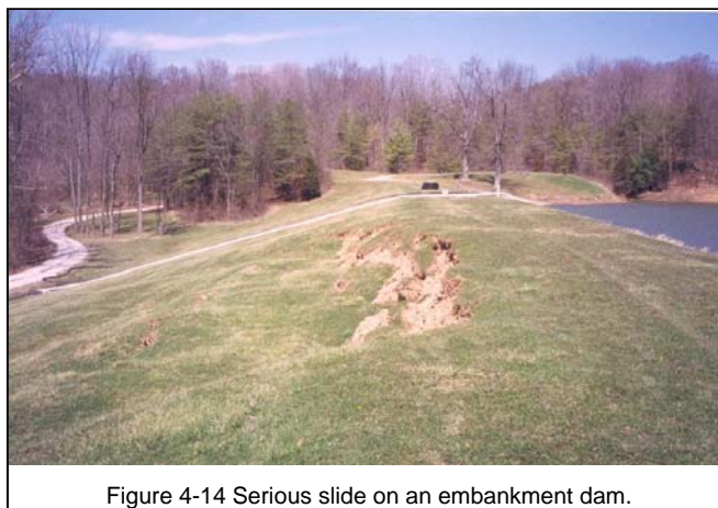
Figure 4-14 Serious slide on an embankment dam.
