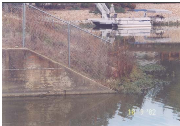
Figure 6-26 Side wall of spillway is spalling.
