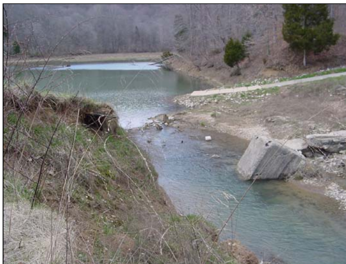
Figure 6-5 This dam's open channel spillway used a concrete control section; note that it failed and was almost totally washed away.
