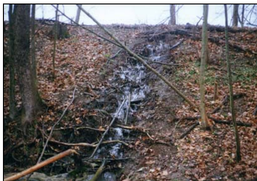
Figure 5-46 Seepage caused by tree roots through the embankment.
