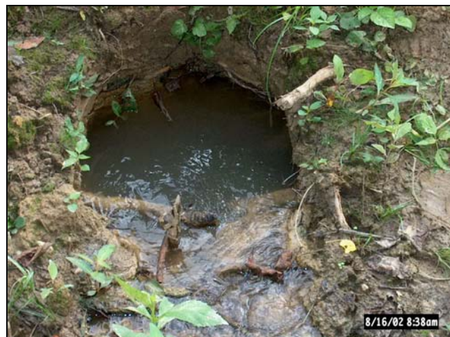
Figure 5-40 Piping with clear discharge may indicate that no additional soil is being removed from the foundation.
