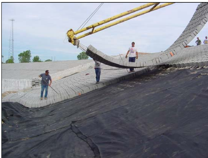
Figure 6-41 Articulating blocks are being placed over a geotextile filter on a dam embankment.
