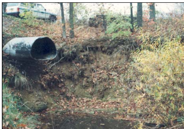
Figure 6-34 The outlet of this spillway has been undermined from the erosive forces of the discharge water.
