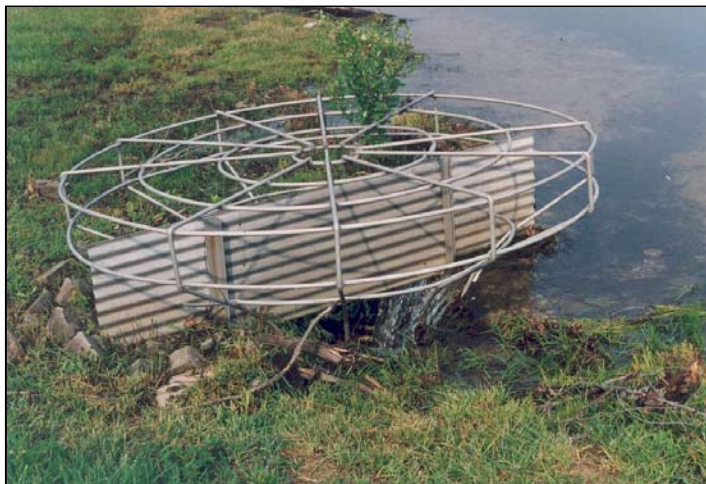
Figure 6-48 Poorly constructed trash rack has openings that are too large at the riser crest.
