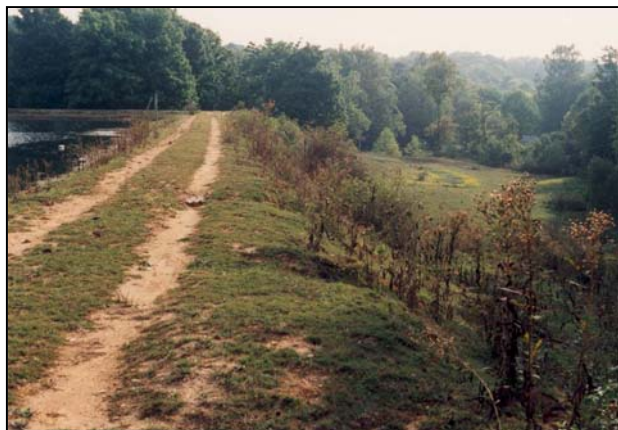
Figure 5-26 Insufficient vegetation on embankment crest and slopes will result in accelerated erosion.
