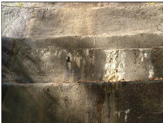
Figure 7-11 Calcium carbonate deposits on the downstream face of a concrete dam as a result of water seepage.
