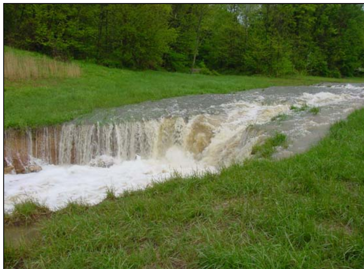
Figure 6-19 Grass lined outlet channel that was not designed for the flows it experienced, resulting in severe erosion.
