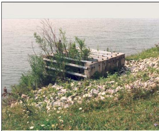
Figure 6-46 Excessive vegetation obstructs this riser structure.
