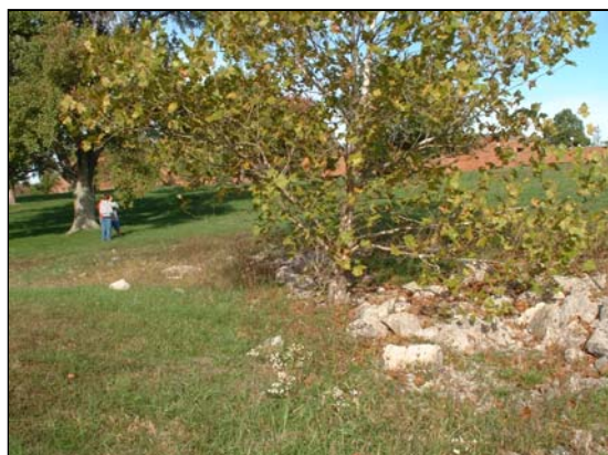
Figure 6-51 Trees growing in emergency spillway.
