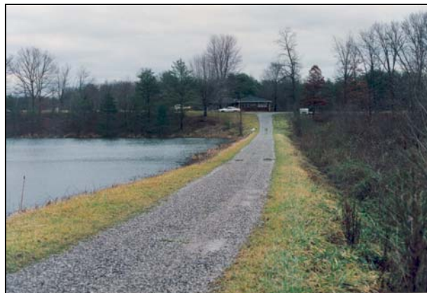
Figure 8-2 This dam has access to and over the embankment, however it may not be able to support heavy equipment.
