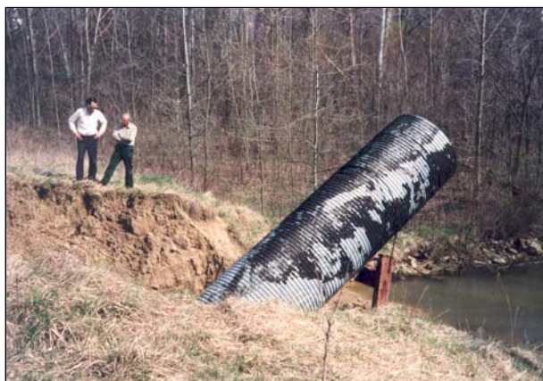
Figure 6-30 Soil erosion under this metal spillway caused the outlet end to settle, resulting in the inlet end tilting upward.
