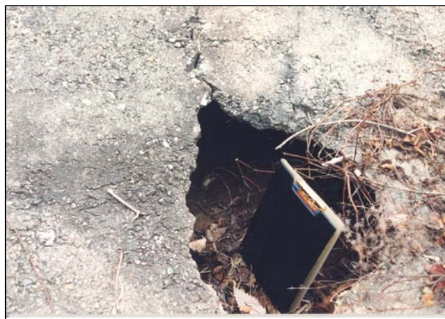
Figure 6-29 Erosion of foundation soil caused this concrete section to fail.
