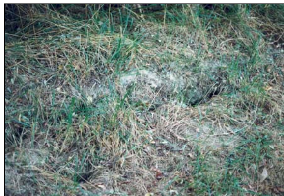
Figure 5-3 Longitudinal cracks on embankment slope.
