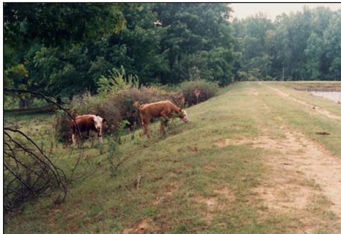
Figure 5-23 Cattle grazing on a dam embankment can lead to erosion problems.
