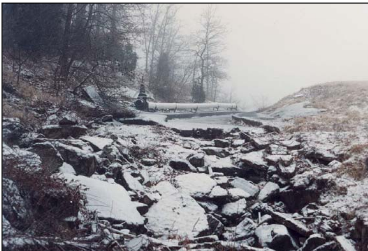
Figure 6-16 Poor spillway lining.
