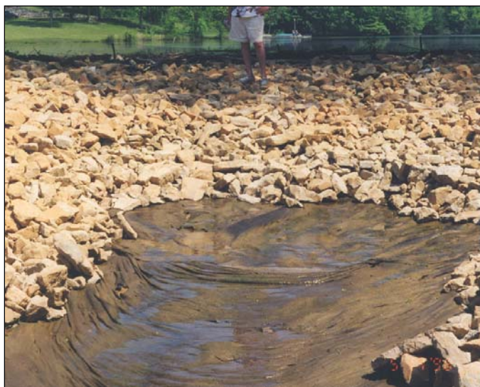
Figure 6-17 Riprap lining was completely washed away during a significant storm event, exposing the geotextile filter.
