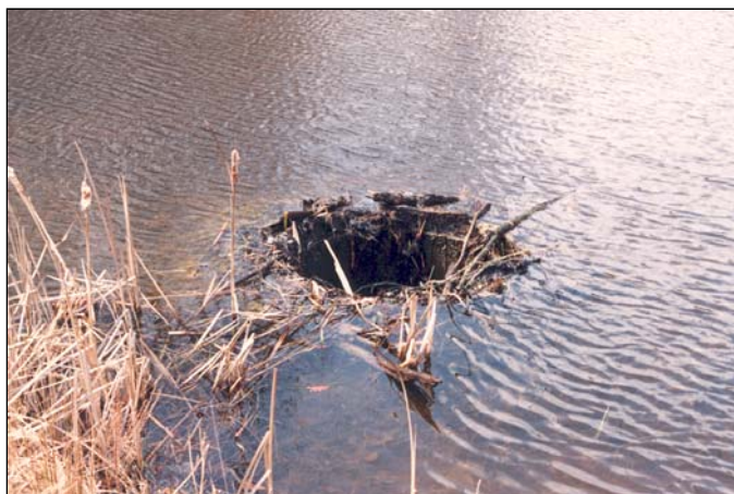
Figure 6-49 Riser lacking a trash rack can clog and cause dam overtopping.
