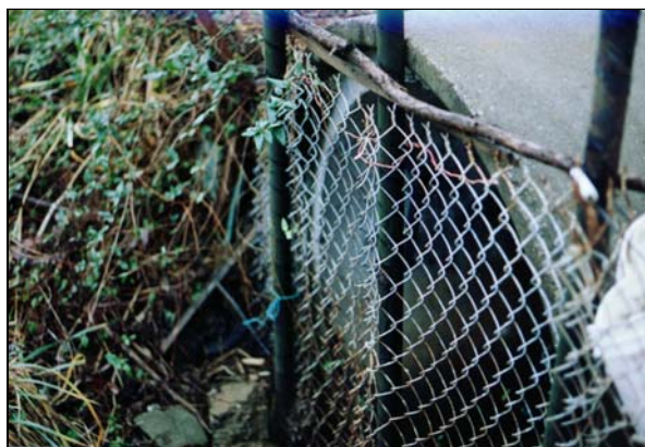
Figure 6-47 Inappropriate trash rack over end of a culvert spillway.
