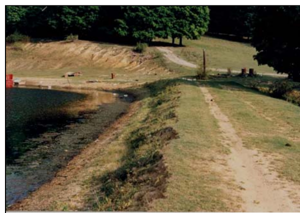
Figure 4-5 Crest problems may be easily seen by sighting along a straight line on the crest.
