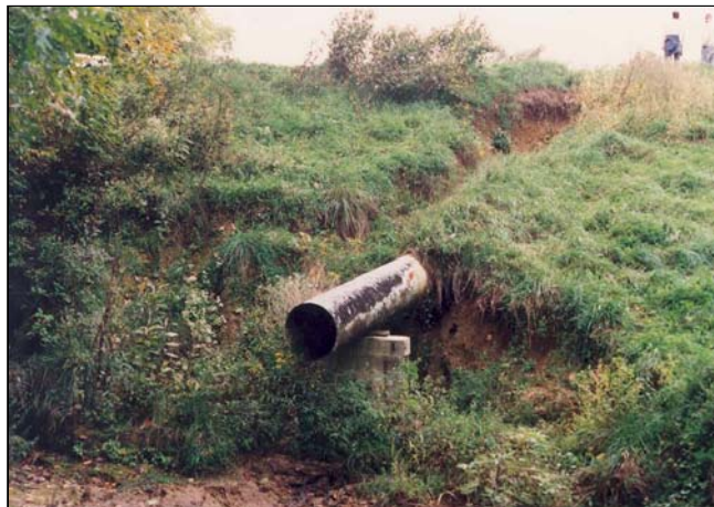
Figure 5-45 Seepage along this spillway conduit has caused piping, sinkholes, and eventual erosion of all the soil over the conduit.
