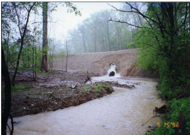
Figure 5-43 Seepage along the spillway in this dam has resulted in piping and a serious leak.
