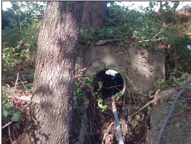
Figure 5-28 A tree is growing over the top of this spillway conduit.
