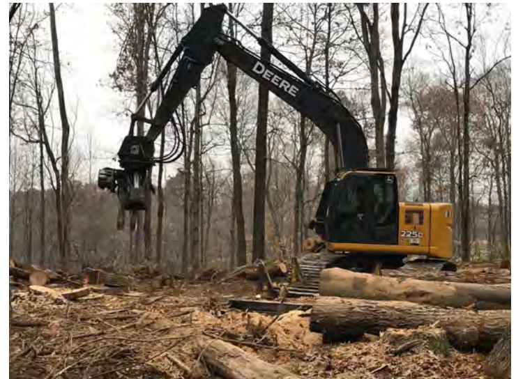
Log landings are where compaction is concentrated on a harvest. Most heavy equipment use the landing and the harvested trees are processed there. Therefore, it is imperative that landings be well-armored and water diverted to stable areas and not onto trails, roads, or bodies of water as the runoff rate is high due to soil compaction.
