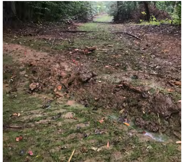
This skid trail has been closed out properly, with waterbars diverting flow off the trail and seeded to expedite growth of vegetation that will stabilize the soil.
