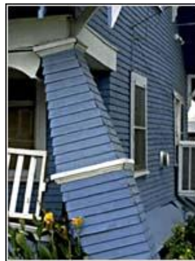
Figure 3-6 Earthquake Damaged Porch
