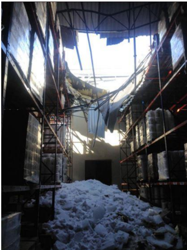
Figure 3-24 Roof Collapse at Performance Foods
