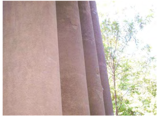
LOOKING N AT SPALLS, DELAMS ON PIER 3 COLUMNS
