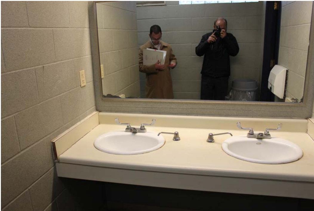
The mirrors are mounted at a non-compliant height. They must be at 40" max.
